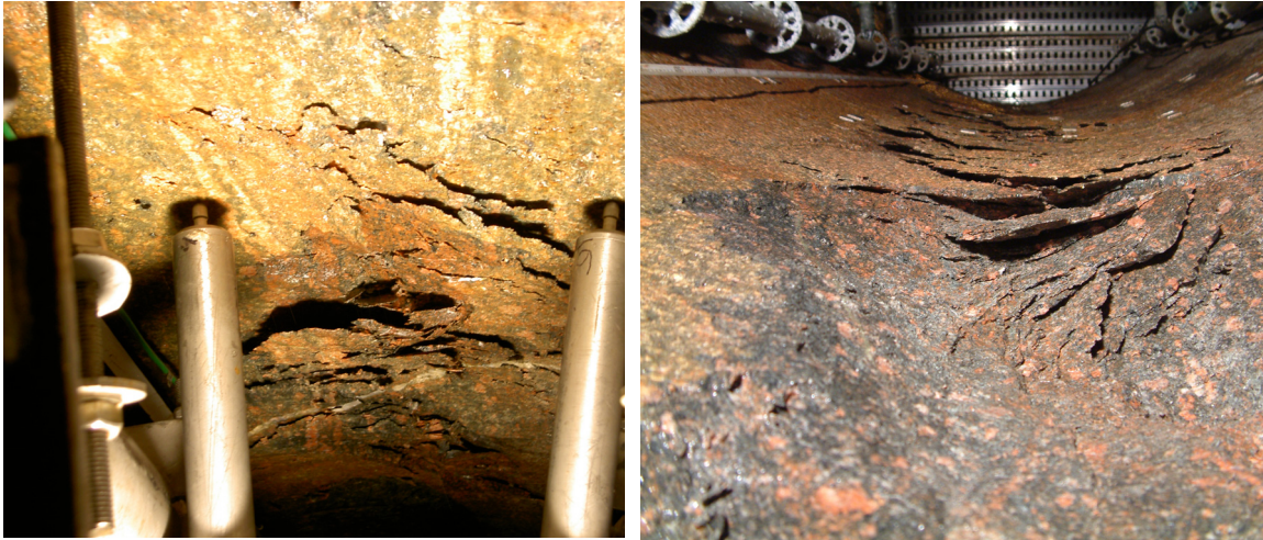
Figure 3-3 Left: the spalling notch propagating downwards and just passing one of the instrument levels where displacement measurements are done by LVDT transducers. Right: Photograph taken from the bottom of the hole and upwards during the removal of the slabs. The different layers of slabs formed are clearly visible as well as the quite smooth surface of the notch that remains after removal of all the slabs.
