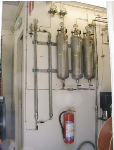
Photo 4. Pressure vessels for test valve, packers and injection.
