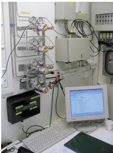
Photo 3. Computer room, displays and gas regulators.
