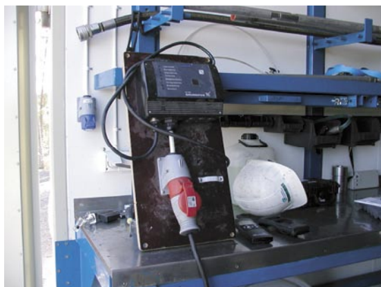
Photo 6. Control board of the pump with remote control.
