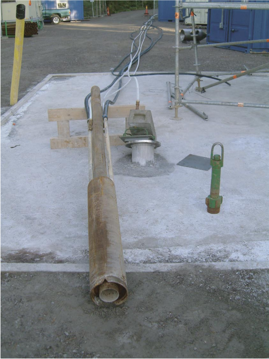
Figure 5-9. The air-lift pumping system.
