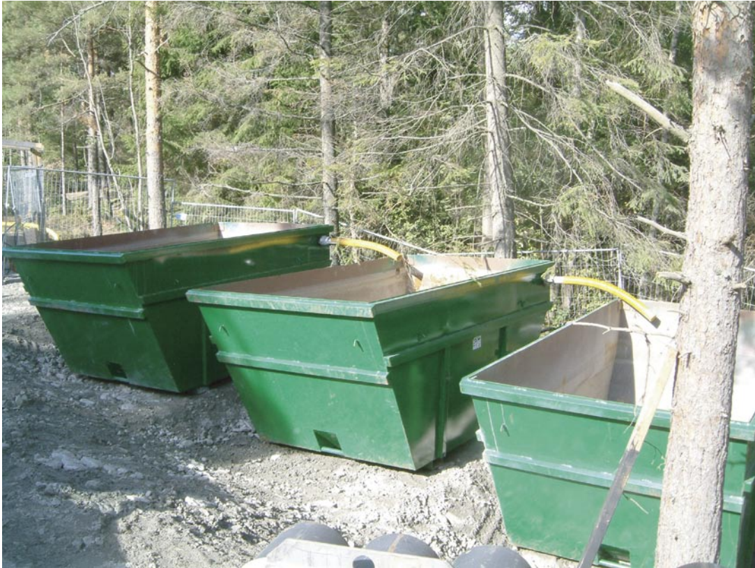
Figure 5-10. The flushing water discharge containers. The sludge and cuttings are allowed to settle in the containers.
