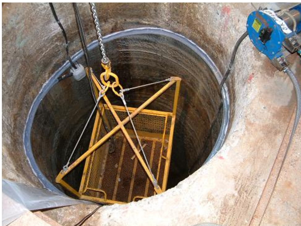
Figure 3-1. Deposition hole DA3147G01 with the circular drain and small plastic container (greyish)
