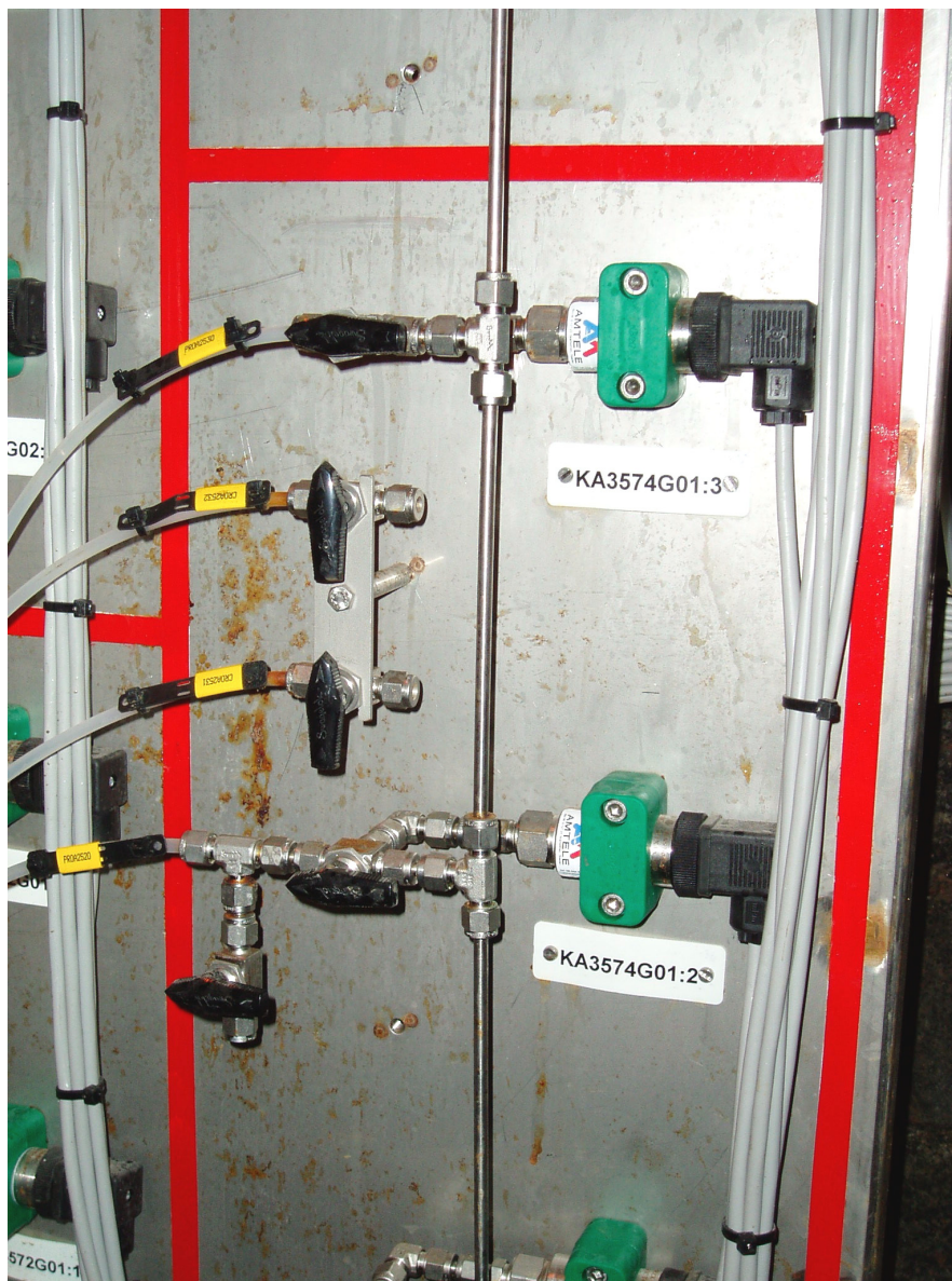
Figure 4-2 Pressure transducers connections
