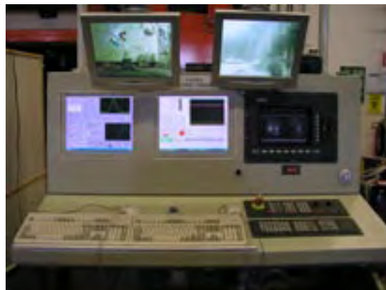
Figure 6-4. Control console for EBW system.
