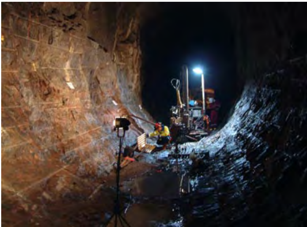
Figure 10-1. The new Apse tunnel at the Äspö HRL excavated during the summer of 2003 by controlled drill-and-blast.
