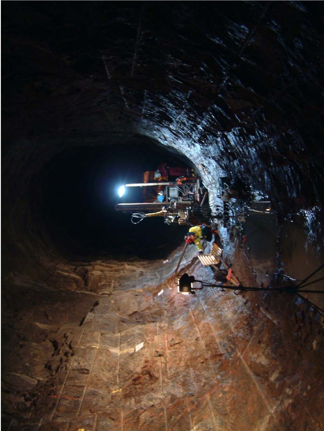
Figure 6. General view from about ch. 75 to 60m. Note accumulation of water in invert and from lower walls, where J_w = 0.66 was the most frequent character logged.
