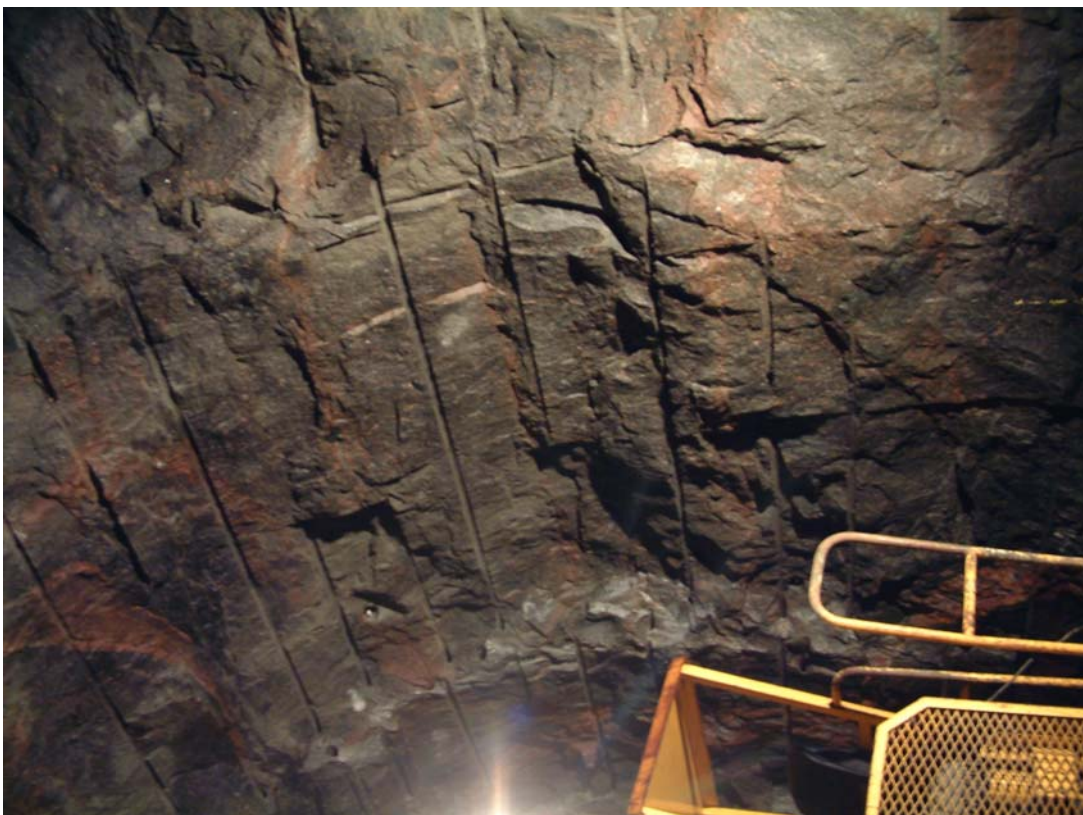
Figure 2. Contrasting quality due to jointing and tangential stress effect: few half-rounds visible on left wall (38 to 46m approx.), excellent arch (45-49m approx.).
