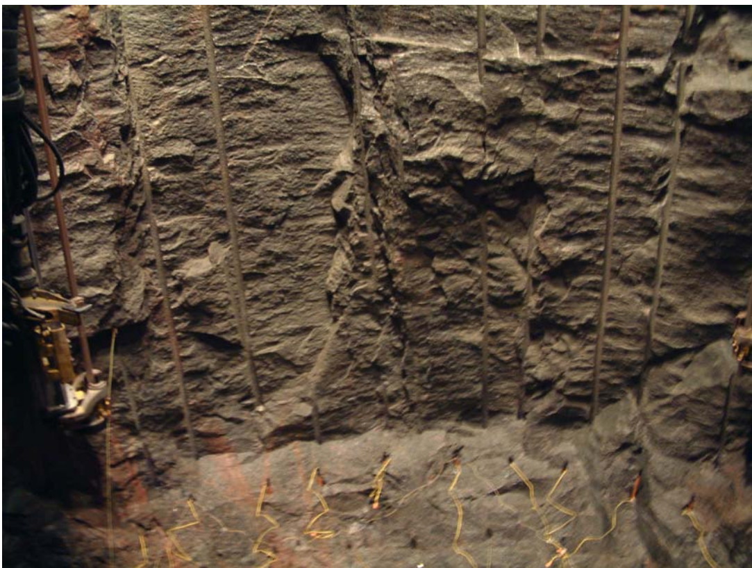
Figure 1. Preparations for blasting with the face at 67m. Note tangential stress effects in arch, and lack of half-rounds in right wall.
