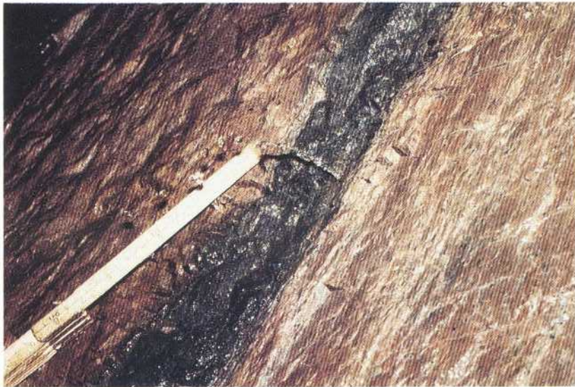
Point leakage ( √ ) from crushed amphibolite plate parallel to the schistosity. The amphibolite is surrounded by leptite. 2/222
