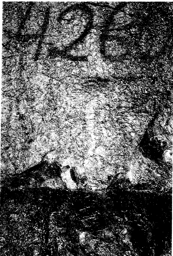
Detail of 5 m long drapery leakage (v-∇) from steep fissure parallel to the tunnel, and in the contact to a crush zone. 4/260
