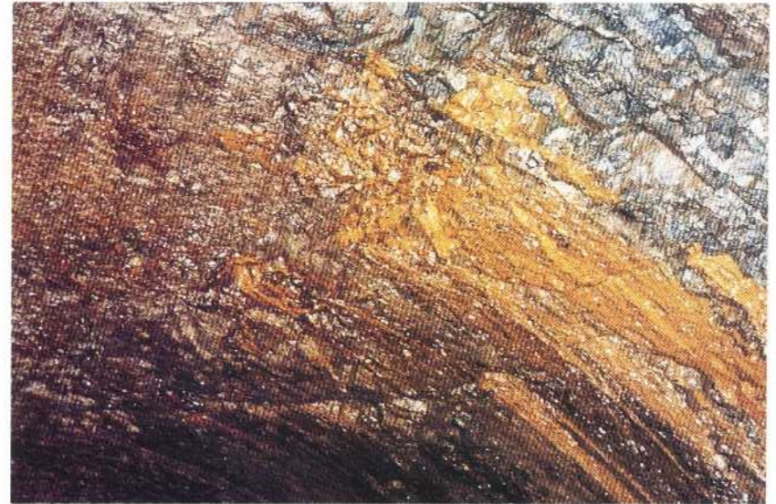
Crush zone with diffuse leakages from the roof and limonite deposition in leptite. 0/435
