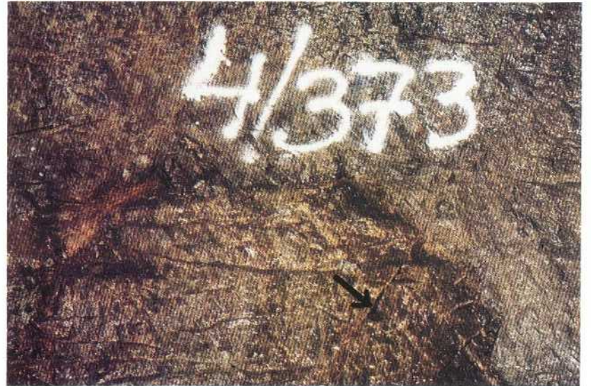
Point leakages (∇) from the schistosity intersected by cracks in granite gneiss. 4/373
