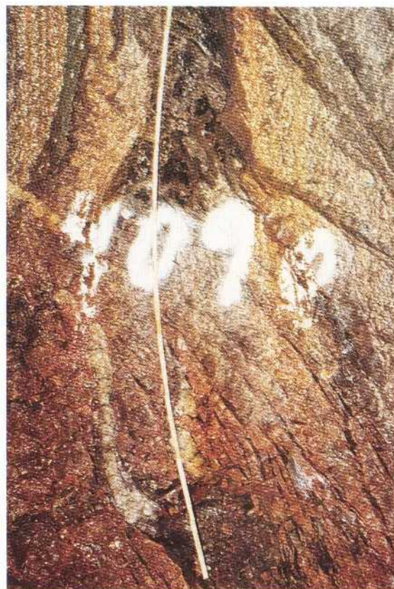
Several point leakages (v-∇) in an irregular crush zone in granite gneiss in connection to amphibolite. 4/090
