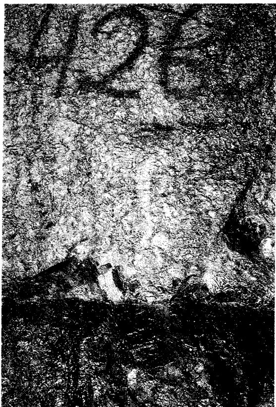
Detail of 5 m long drapery leakage (v-∇) from steep fissure parallel to the tunnel, and in the contact to a crush zone. 4/260
