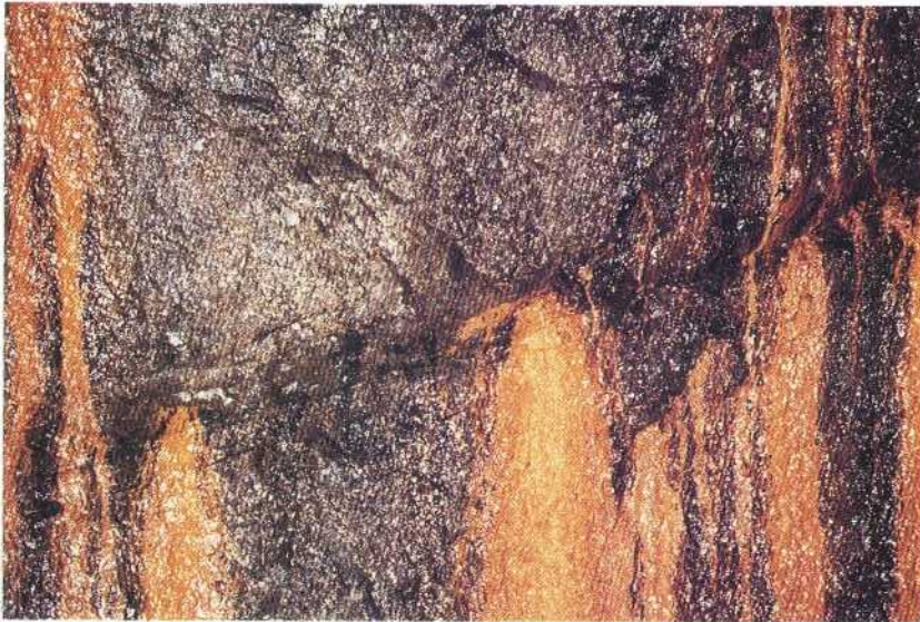
Extensive point leakages (V-V) from steep fissure parallel to the tunnel in leptite. 0/316
