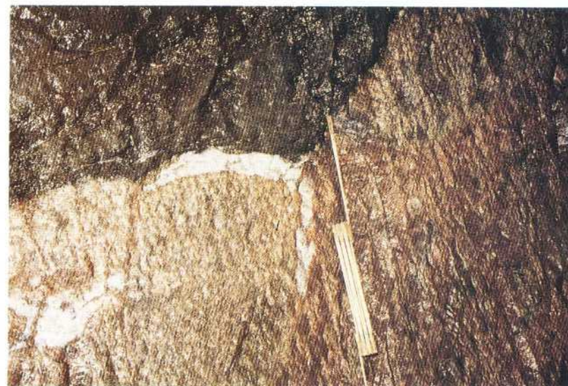
Minor point leakages in the contacts between amphibolite, granite gneiss (left) and leptite (right). 0/870
