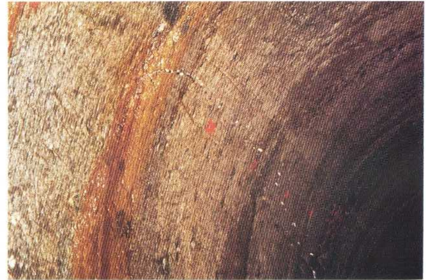
Strong point leakage (2 l/min) from fissure in thin amphibolite not parallel to the schistosity, developed in the surrounding leptite. 2/220
