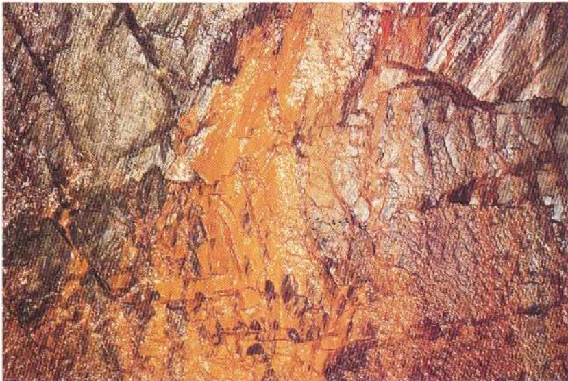
Several diffuse leakages with extensive limonite deposits in crush zone in leptite. 4/226
