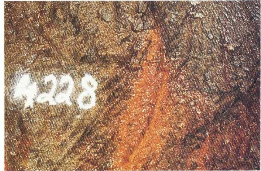
Drapery leakage (∇) 0,5 m long from fissure not parallell to the schistosity in crushed leptite. 4/228
