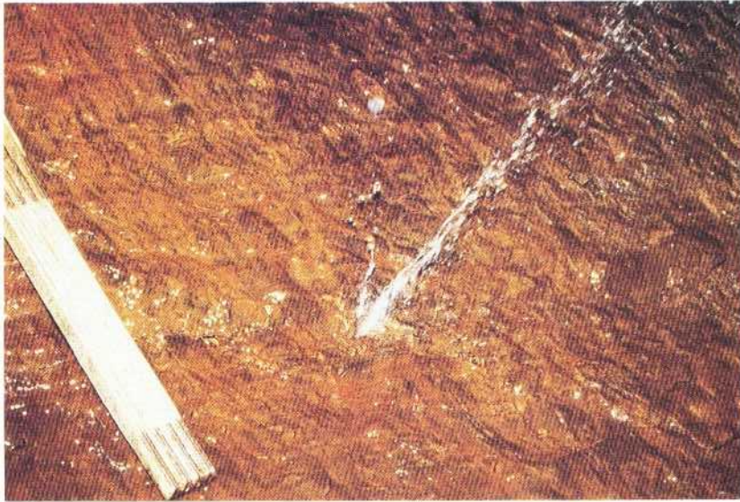
Strong point leakage ( √ ) from crack in crush zone in leptite. 2/272
