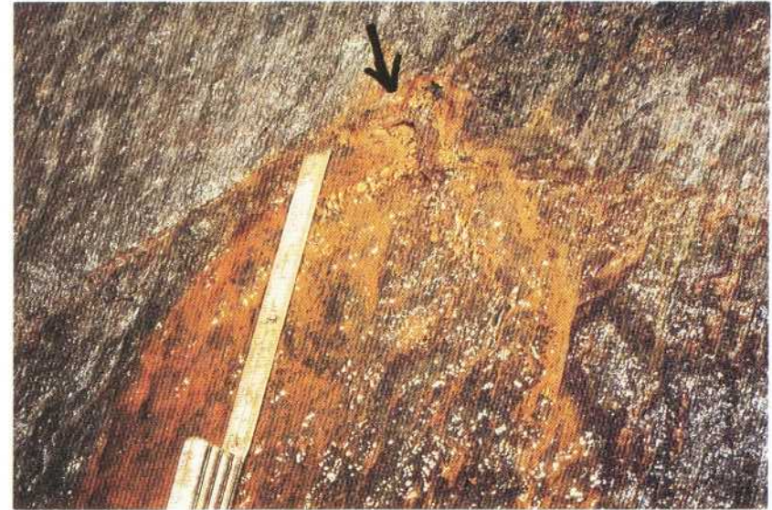
Point leakage ( √ ) from fissure perpendicular to the schistosity in leptite. 2/665
