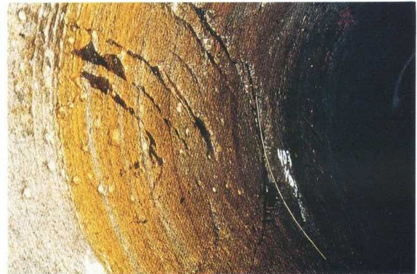
Several point leakages (v-∇) from steep cracks parallell to the tunnel in leptite. 4/030
