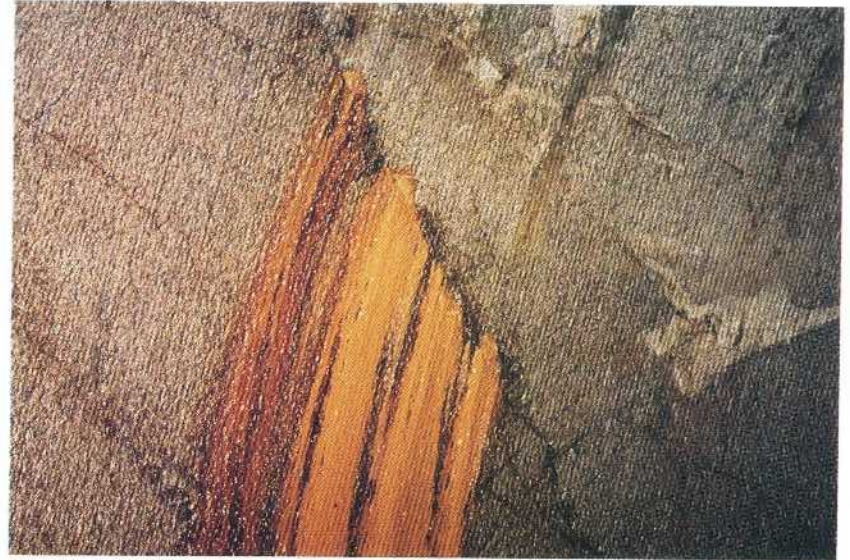
One meter long drapery leakage (V) from a crack in granite gneiss. 1/090
