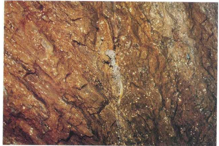
Strong point leakage (V) from fissure parallel to the schistosity in thin amphibolite plate in granite gneiss.
