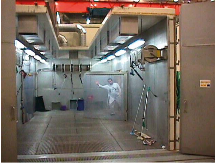
Figure 8-3. Example of high pressure water decontamination facility at Oskarshamn.
