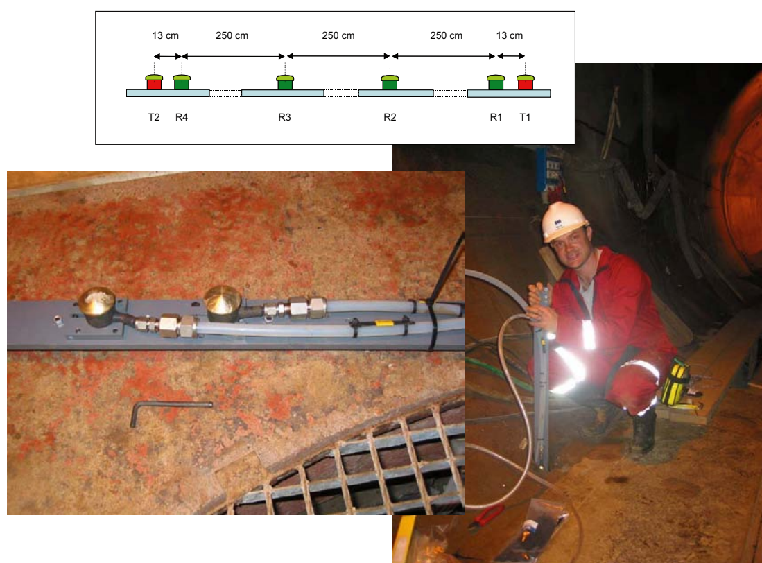
Figure A2-1. Top: Schematic diagram of the locations of all transducers on a single frame. Left: Photo of a section of the transducer assembly. Right: Transducer assembly during installation.
