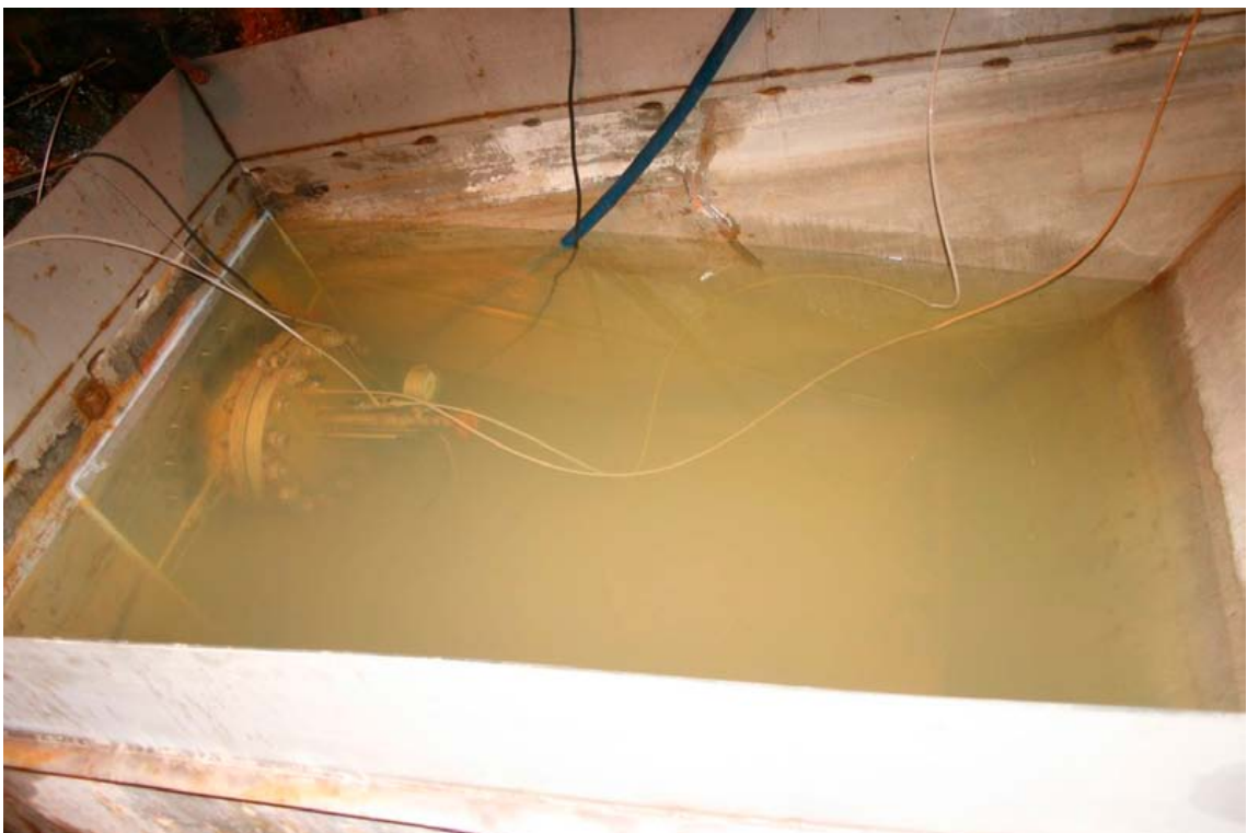
Figure 2-5. Photograph from above the transfer tank showing the borehole flange below the waterline.
