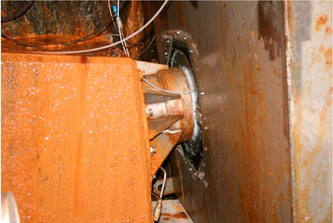
Figure 2-4. Photograph of transfer tank to flange coupling.
