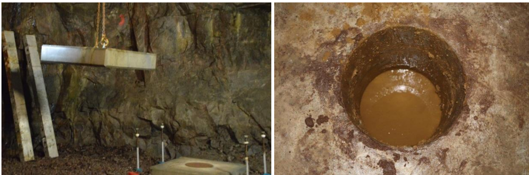
Figure 4-1. The concrete lid is removed (left image). After removing the top seal, water was observed in the installation hole.
