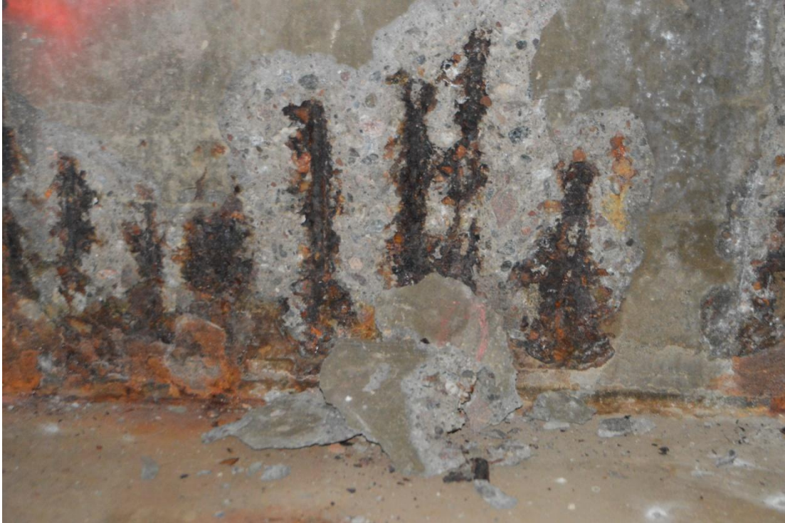
Figure 1-1. Concrete spalling due to corrosion of reinforcement bars.
