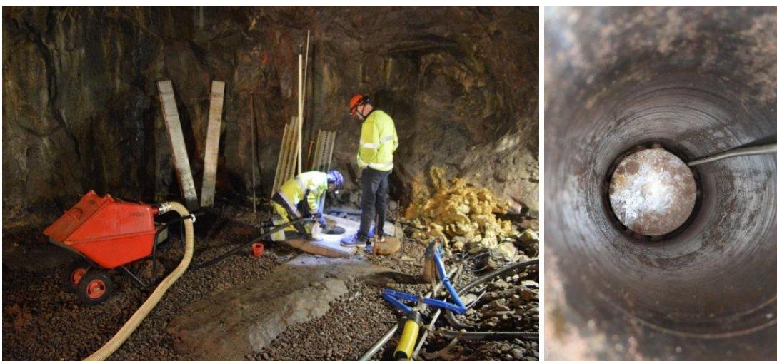
Figure 4-2. Cleansing of the sand-filled slit between the concrete cylinders and the wall of the installation hole.
