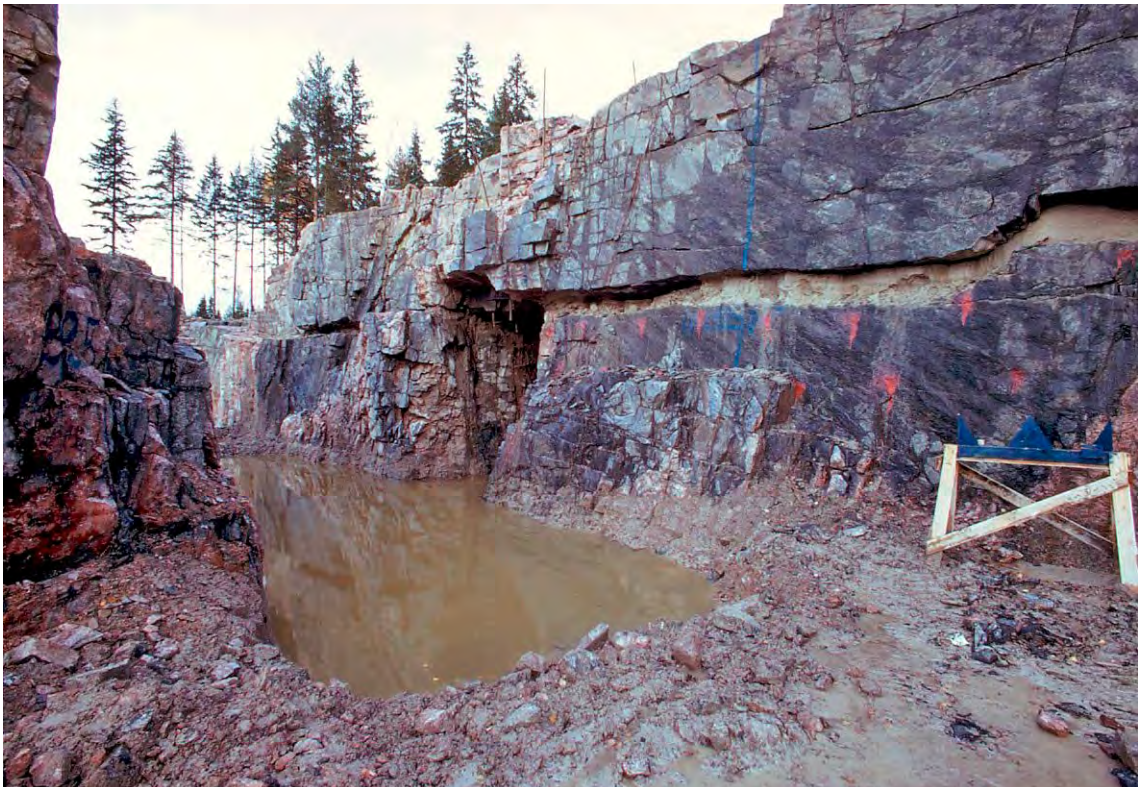
Figure 4-16. Shaft wall along a water reservoir during the foundation of the nuclear power plant. A sediment-filled sheet joint with an aperture of approximately 0.5 m runs along the shaft. Photography by G. Hansson.
