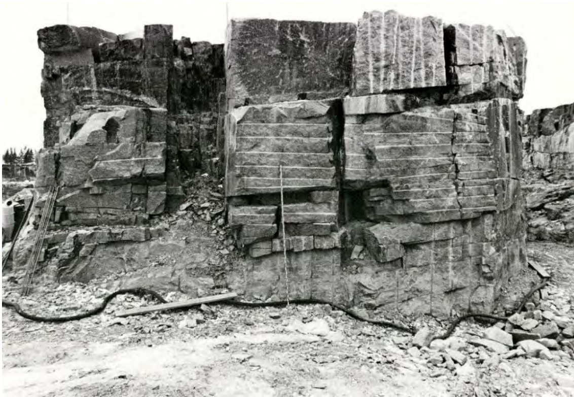
Figure 4-19. Shaft wall at reactor block 3, which displays a vertically dipping fracture zone (oriented 040^{\circ}/90^{\circ} ) intersected by a set of sheet joints. Length of the levelling staff is 4 m. From Carlsson (1979). Photography by G. Hansson.
