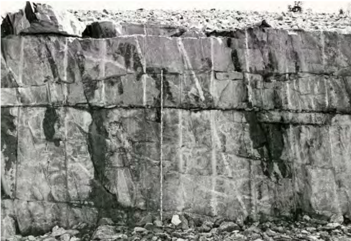
Figure 4-30. Examples from shaft walls along the inlet channel that illustrate the local variability in the fracture intensity in the near-surface bedrock. The distance between the two localities is ca 20 m. Length of the levelling staff is 4 m. From Carlsson (1979). Photography by G. Hansson.
