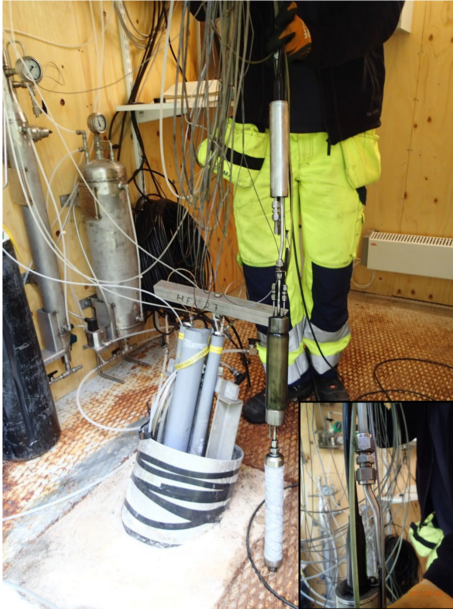
Figure 2-4. The pumping equipment (GEOPUMP UV-45) used for pumping in wide standpipes. The equipment consists of a filter and a pump connected to the mini-packer. The small diameter plastic hose is used for expanding the packer and the plastic hose connected to the pump is the pumping hose (enclosed picture right lower corner).
