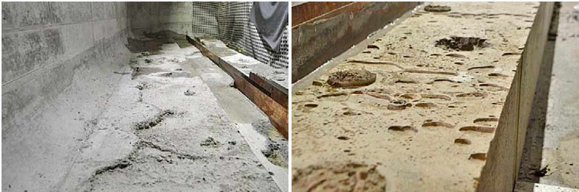
Figure 5-12. Images showing details of different types of imperfections in the base slab.
