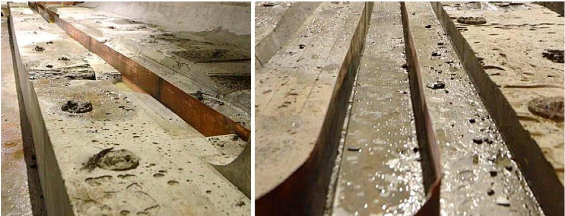
Figure 5-15. The joint seal mounted in the base slab at the position of the future section 2 of the concrete structure.
