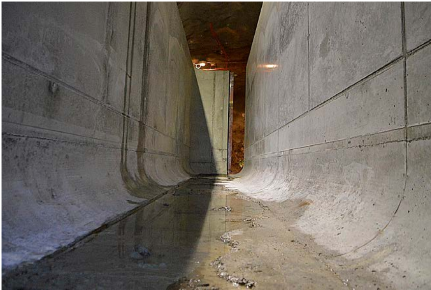
Figure 6-6. The interior of the concrete structure with section 2 to the left and section 1 to the right. Note the rather large amount of water on the base slab caused by ground water dripping from tunnel roof.
