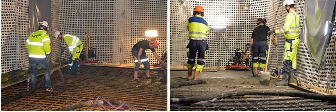
Figure 4-3. Casting of the concrete slab has started (left image) and casting and trowelling of the topmost layer (right image).
