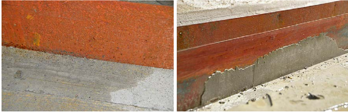
Figure 5-16. Images showing the adhesion between the concrete and the joint seal.
