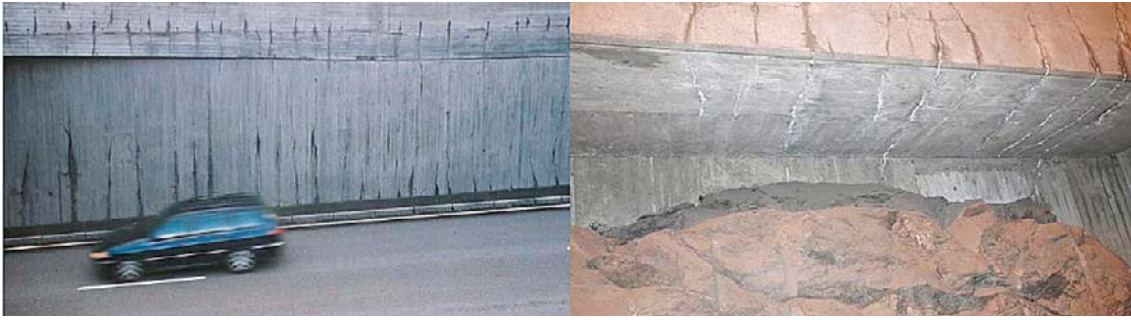
Figure A-1. Early age cracks in retaining walls, left picture: Anders Hösthagen, BOSTEK, right picture: Jonatan Paulsson-Tralla, BOSTEK.
