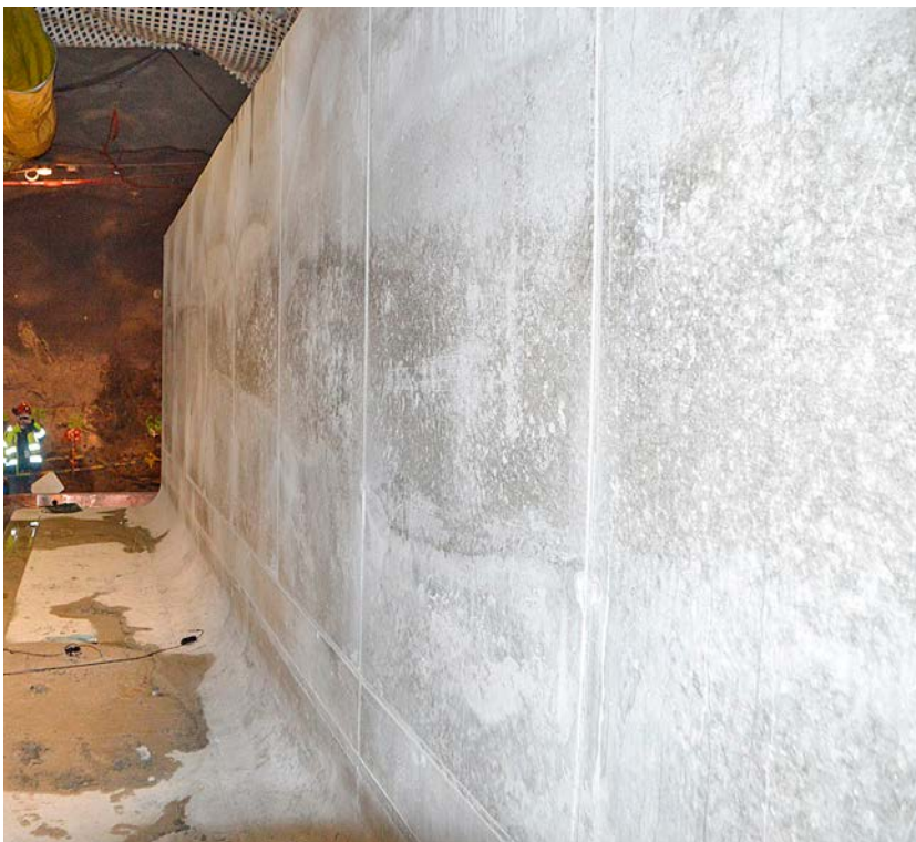
Figure 5-13. The surface of the walls were smooth and only a very few imperfections were detected. Also, the concrete was dense and homogeneous in spite of the encountered problems.
