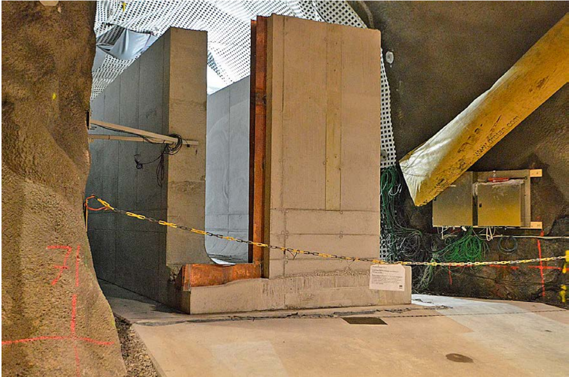
Figure 6-5. An overview image of section 1 (left part) and section 2 (right part). The horizontal joint seal in the base slab and the vertical joint seal in the wall of section 2 are clearly visible.
