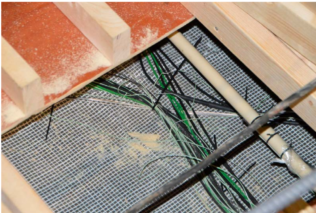
Figure 5-4. Cables from the sensors placed on the plastic foil on top of the concrete slab. Note that the cables are loose and unprotected.
