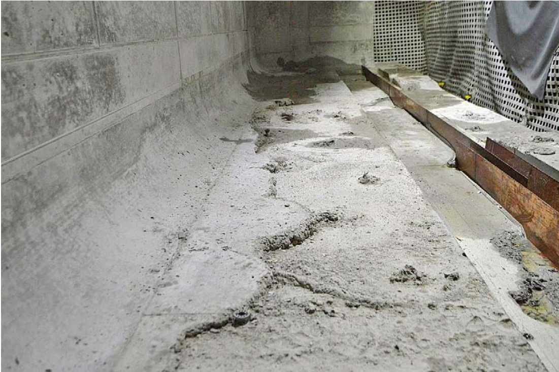
Figure 5-14. Image showing the complete filling of the fillet between the wall and the base slab of section 1. However, in this image it is also shown that the concrete has not entirely covered the surface of the base slab due to low mobility.
