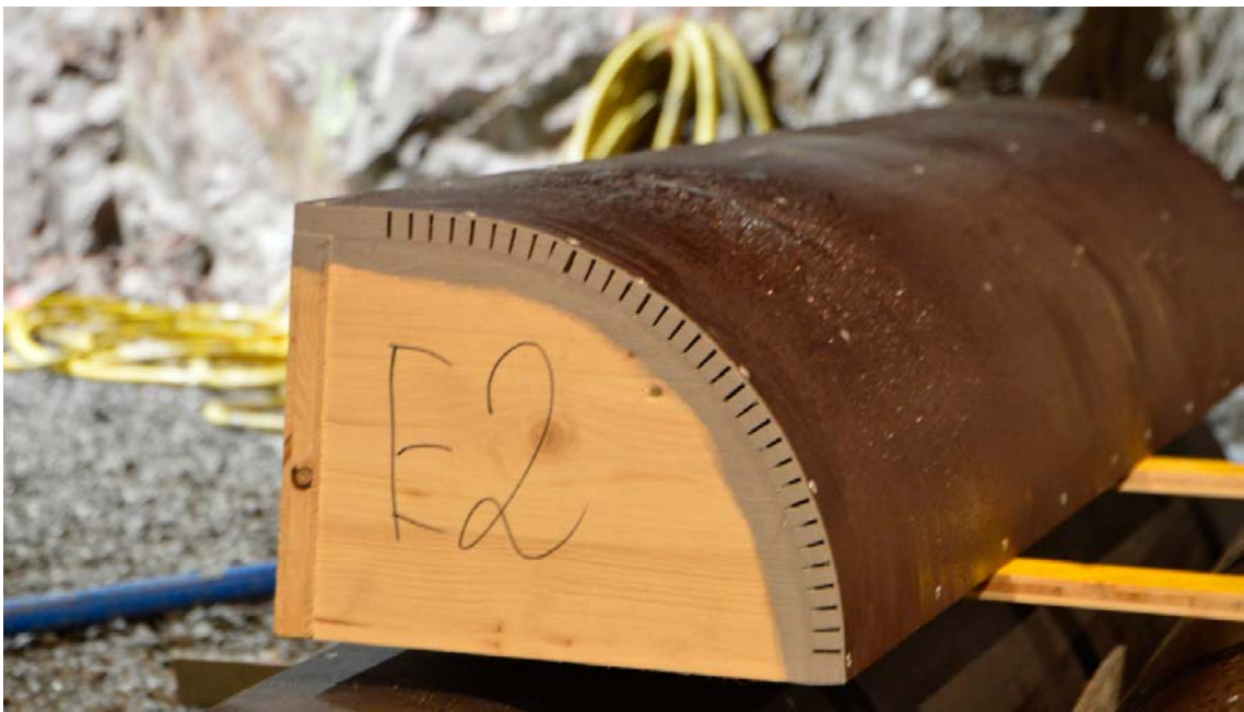
Figure 5-2. The part of the formwork used to shape the radius between the base slab and the wall of section 1.
