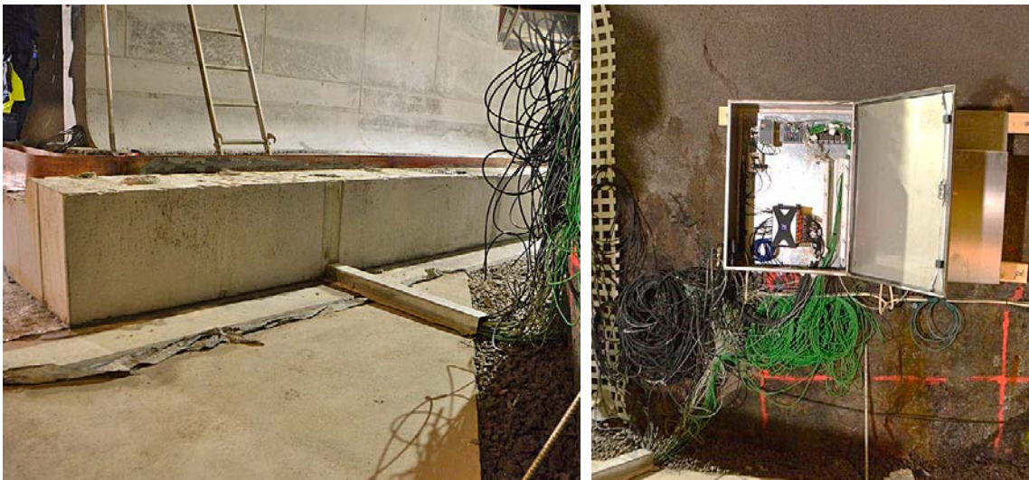
Figure 3-10. All cables from the different sensors were collected into one bundle (left image) and signals were collected in the control cabinet (right image).
