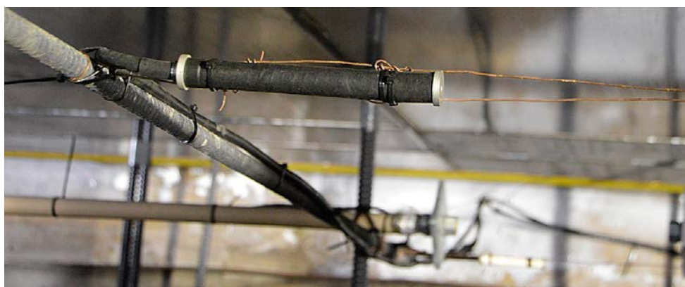
Figure 6-2. Sensor suspended on the system of rods inside the formwork of the wall of section 2.
