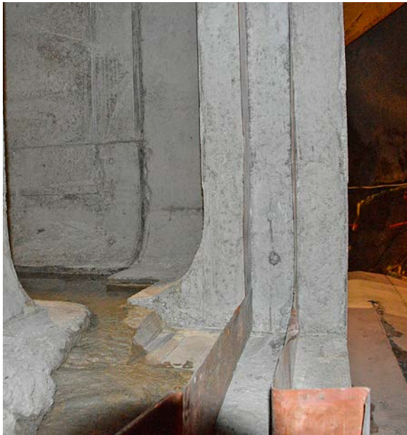
Figure 6-7. Form filling in the fillet between section 2 and the base slab of section 1. This image also shows that the filling between the vertical joint seals in section 2 is complete.
