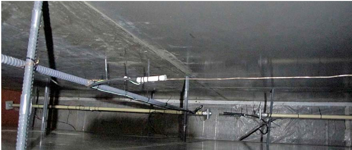
Figure 5-3. Sensors suspended on the system of rods inside the form work of the wall of section 1.
