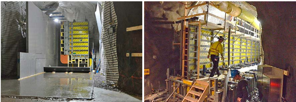
Figure 5-1. The formwork under construction (left image) and ready just prior to casting (right image).
