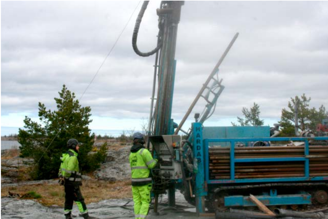
Figure 3-1. The HARDAR 5000H drilling machine at drill site HFM45. The automatic rod handling system has grabbed a new drill rod that is ready to be positioned as soon as drilling stops.
