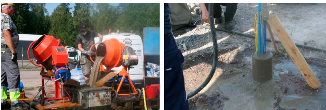
Figure A1-3. To the left: The completed cement paste was poured into a screw pump that pressed the paste into the pipe so that the borehole was filled from bottom and upwards. To the right: As the cement rose in the borehole, the water column was lifted at TOC, meaning that the entire borehole had been injected.
