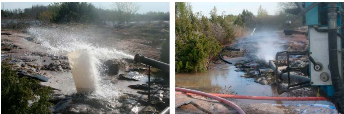
Figure 5-10. Left: In HFM45 the accumulated water inflow increased to c 100 L/min at the complete borehole length, 200 m. Right: In HFM46 the accumulated water inflow increased to 400 L/min during air flushing at the final drilling length at 200 m.
