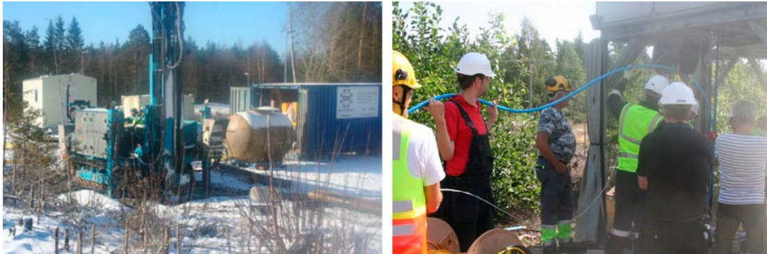
Figure A1-1. Left: When performing drilling of HFM42, the ground surface was covered with snow (April 2018). Right: Installations in HFM42 from a two-stage podium. On August 8th the temperature had raised to 30° C.
