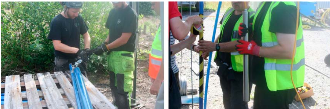
Figure A1-2. Left: A steel wire was attached to the steel pipe (grouting tube) and welded together with a bull-nose aimed to protect the ends of the two fibre cables. Right: The two fibre cables were fastened to a rod with cable ties for each m. As the pipe was lowered into the borehole, three geophones were mounted at 188 m, 74 m, and 6.5 m borehole length.
