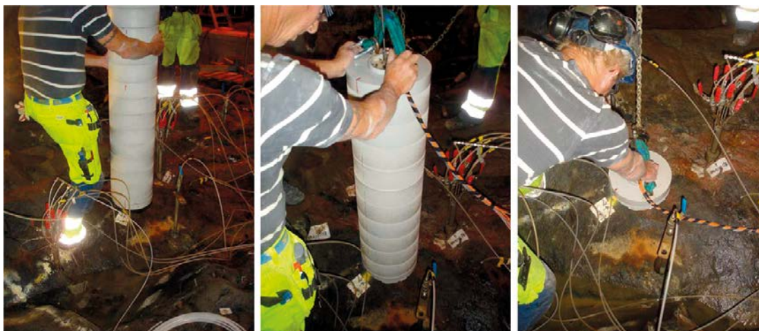
Figure 2-11. Installation of the bentonite blocks in KO0017G01. Photographs are reproduced from the task description (Vidstrand et al. 2017).
