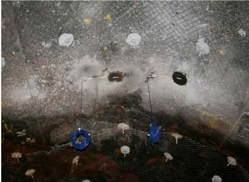
Figure 3-5. Five pressure sensors were installed in the ceiling above the deposition hole.
