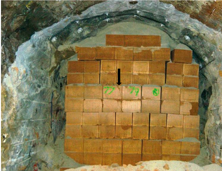
Figure 4-8. The block stack at the vertical section 6 (see Figure 3-10) just before reaching the deposition hole (at the lower part) and close to the midpoint over the deposition hole at the top of the block stack.
