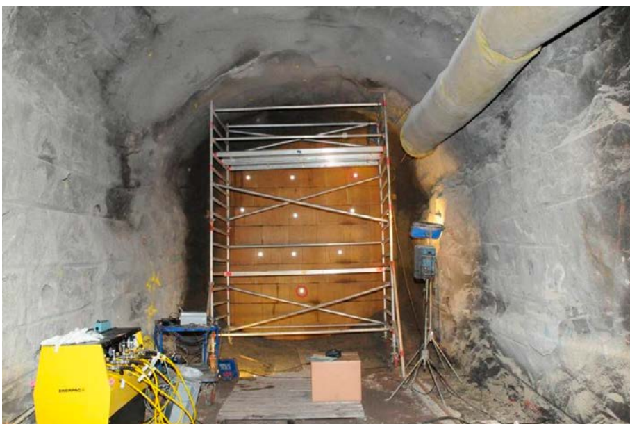
Figure 3-8. The block positions were determined with reflectors at ten points at the end of the block stack.
