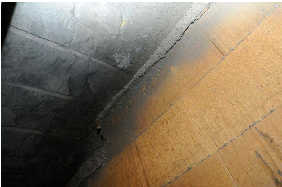
Figure 4-6. The pellet filling on top of the block stack had been pushed out about 40 to 50 mm. The outermost part of the pellet filling was pre-wetted, during the BST construction in order to keep loose dry pellet materials from falling out of the downstream face. The result of this is that the pellets stick to the ceiling and when extruded by internal deformation, do so as a plastic mass.
