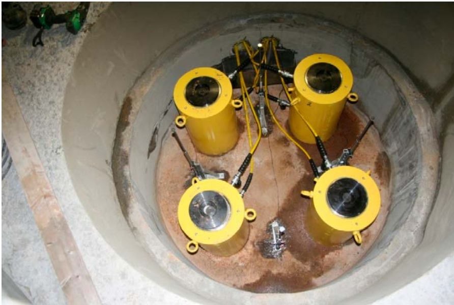
Figure 3-1. The four hydraulic jacks and the four displacement sensors installed in the artificial deposition hole
