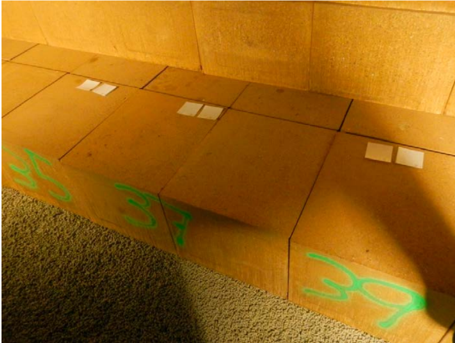
Figure 3-7. The pressure indicators were placed between the backfill blocks at selected positions. Two sensors with different measuring range were placed on each block.
