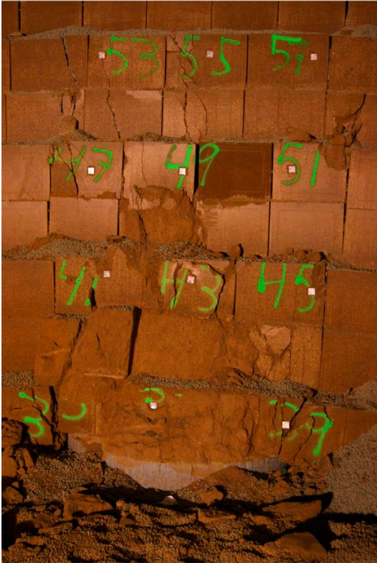
Figure 4-18. Extensive shear surfaces and fractures in the blocks immediately above the deposition hole.
