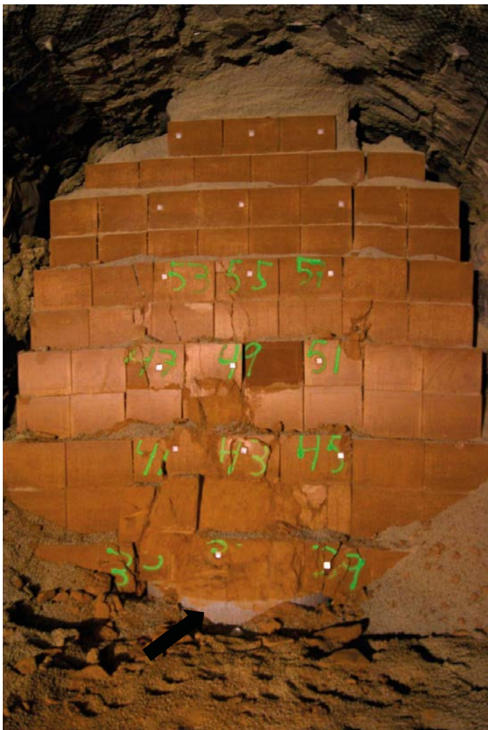
Figure 4-17. Overview of the block stack above the deposition hole with buffer showing at the base (black arrow). The shearing of backfill blocks is mostly to the left of center, while blocks on the right side seem to have moved out into the pellet slot rather than failing.
