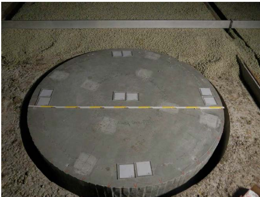
Figure 3-6. Pressure indicators placed on the buffer block.
