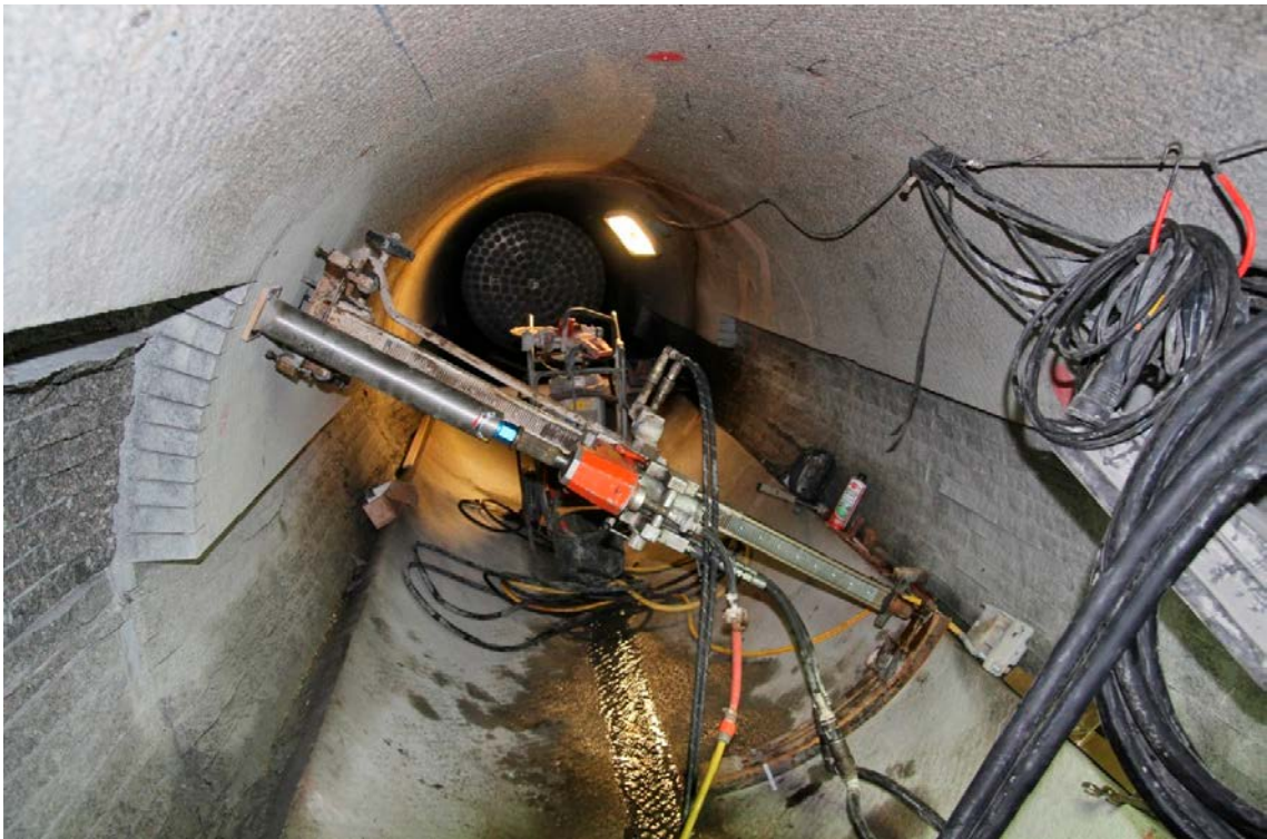
Figure 5-6. Core drilling of 10 m long boreholes inside the MPT test section. The picture also visualises the cable notches. Note that the Supercontainer vaguely seen at the end of the drift is the concrete dummy used during deposition machine testing; it was removed prior to the main MPT installation.
