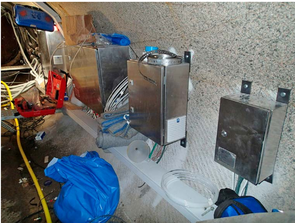
Figure 9-16. Connection cabinets placed on the drift wall immediately outside the plug.
