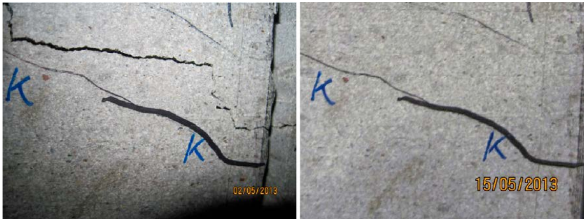
Figure 7-1. To the left, one of the worst drying cracks noted on the distance blocks, several centimetres long and in the order of 1 mm wide. To the right a picture of the same area once the block had been stored for some days in a RH corresponding to its equilibrium state, the closing of the crack is apparent.
