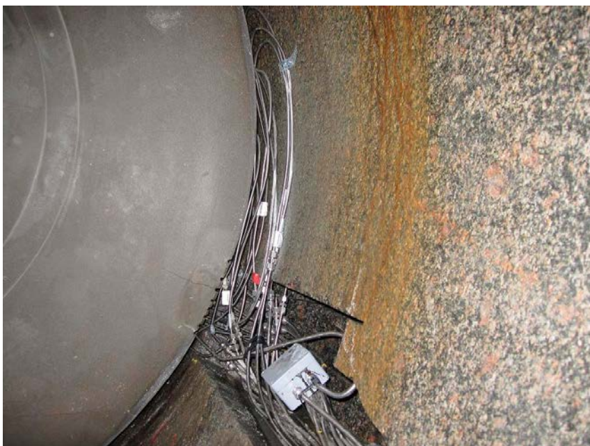
Figure 9-4. One of the sides of the inner distance blocks with all cables connected and the cable block removed.
