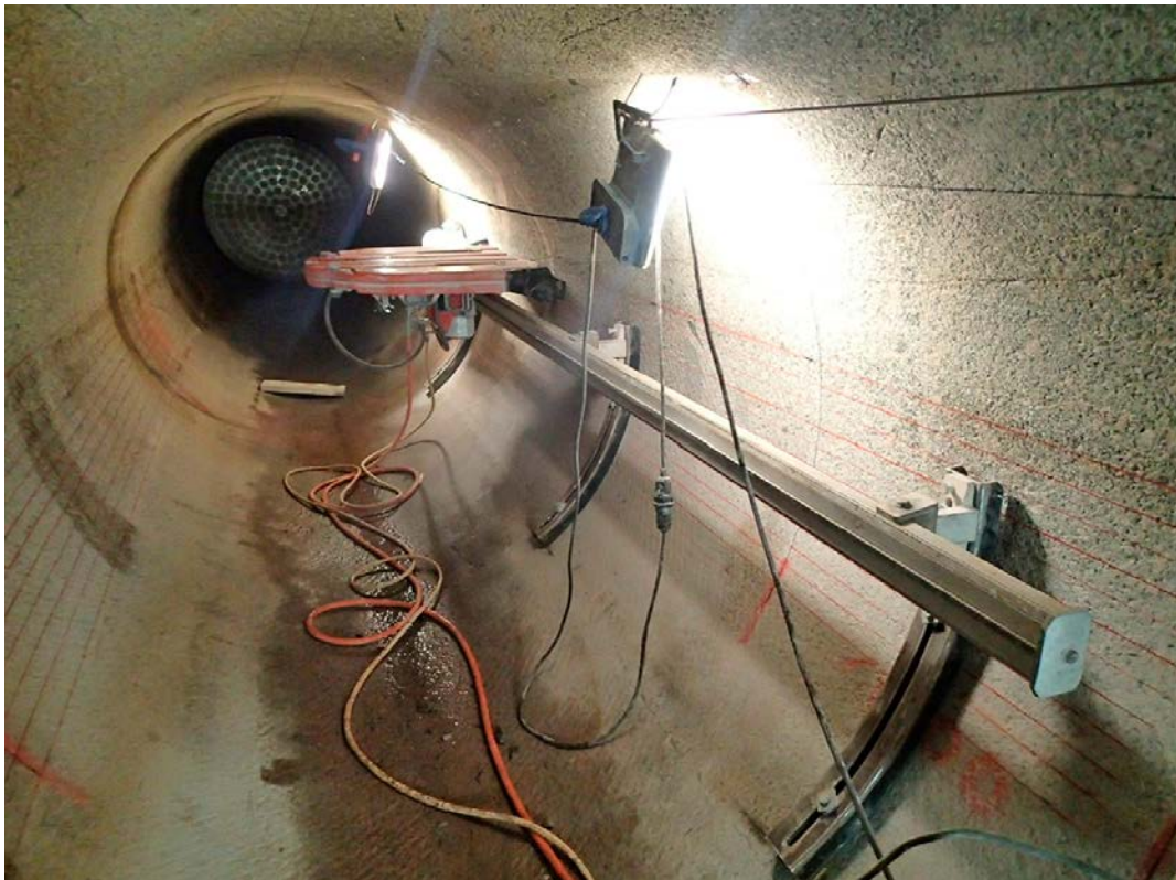
Figure 5-5. Saw fitted on rails with anchorings that allow for cutting of parallel cuts along the drift sides. Slices of rock were later broken off starting at the highest point and continuing downward.
