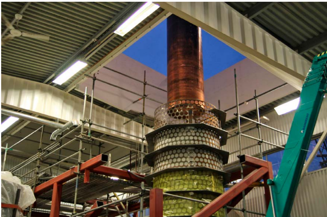
Figure 8-8. Canister being lowered into the Supercontainer. The stiffening plates for straightening the shell can be seen on its outer periphery.
