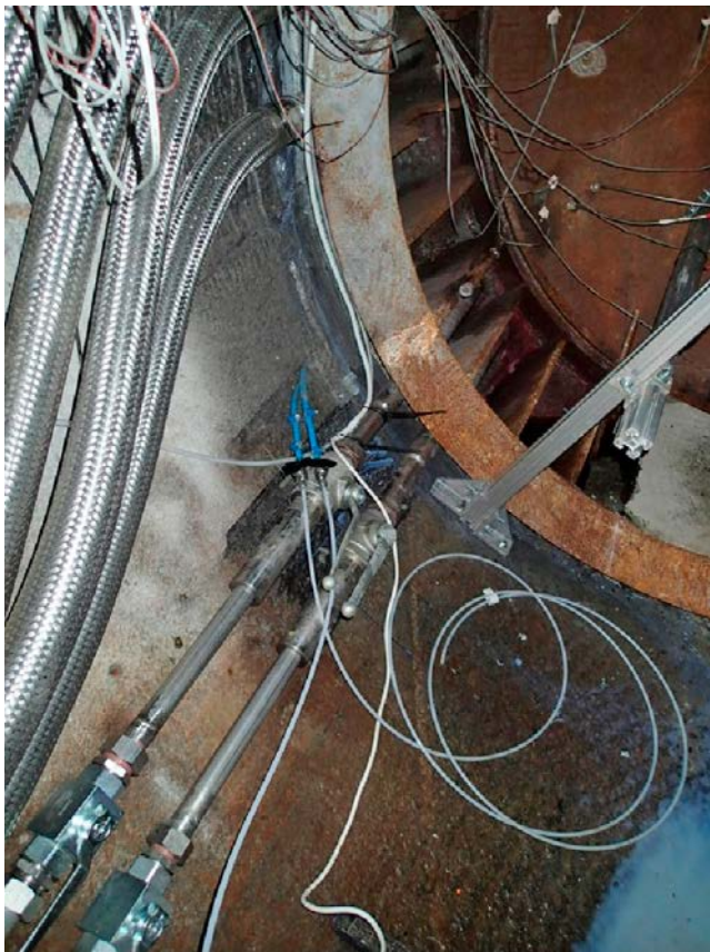
Figure 9-17. Contact grouting in the blue tubes, corresponding to the casting-steel interface. The silica sol seen down to the right is from flushing prior to starting the grouting. The silica sol leaking out at 9 and 4 o'clock was much less.
