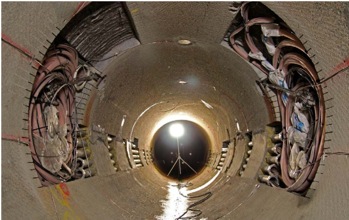
Figure 5-10. The MPT drift prepared for installation, note the partial low-pH casting around the larger pipes. Also visible is the cable storages where tubes and cables are placed during installation.
