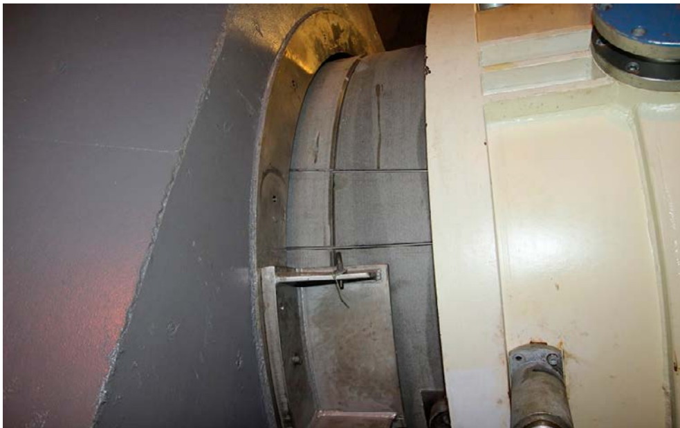
Figure 7-8. Distance block driven in to the drift from the transport tube. The tight fit between the component and drift wall when it is lifted can be seen in the top part of the picture.
