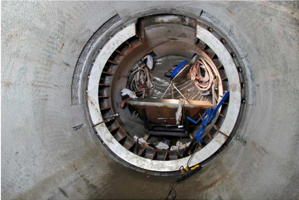
Figure 9-10. Three of the collar segments placed with only the fourth smaller top segment remaining. The plug cap, leaning on its steel support can be seen between the collar and the transition block.
