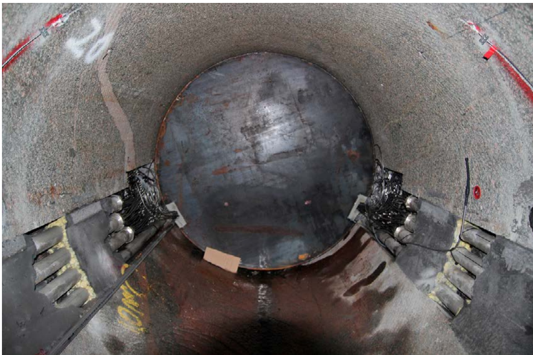
Figure 9-7. Supercontainer positioned in the drift with all its cables pulled. The tight fit between the Supercontainer and drift wall is clearly visible. A small paper has been placed down to the left of the Supercontainer to ensure that the deposition machine will detect the Supercontainer during deposition of the next component.
