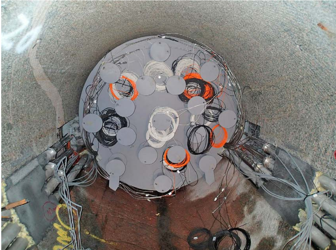
Figure 9-6. Pulling of cables from the Supercontainer to the main piping in the drift walls and to the cable storage, cf. Figure 5-10.
