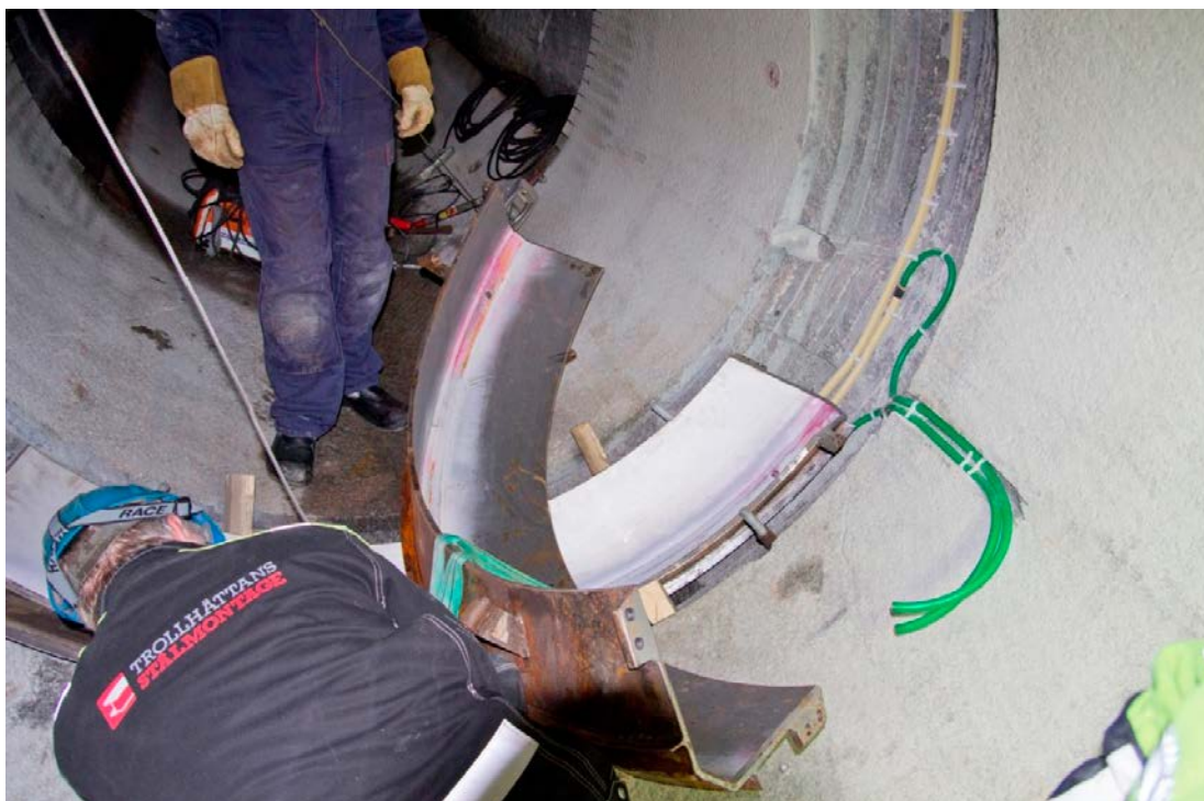
Figure 5-3. Installation of the fastening ring, the contact grouting tube in the rock-casting interface can be seen to the right in the picture.
