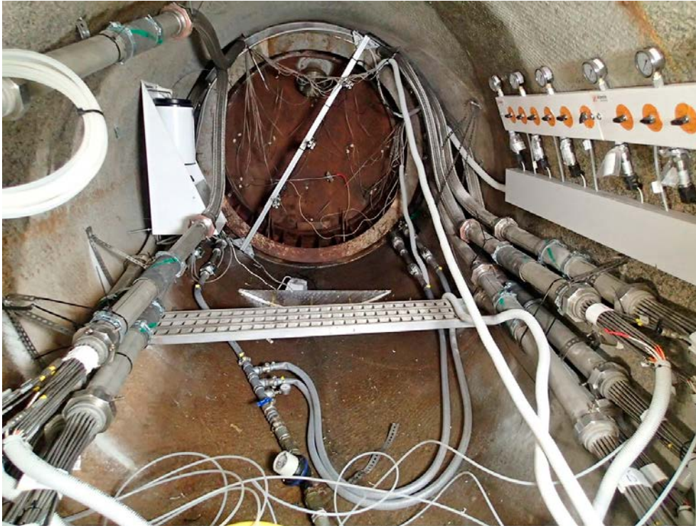
Figure 9-15. Flexible piping and outer 'hedgehogs' with the cabling inside. The picture was taken during the DAWE procedure.
