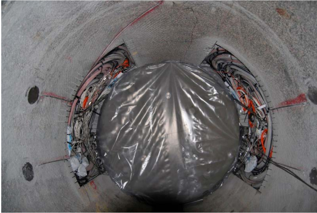
Figure 9-9. Transition block deposited and protected by plastic film awaiting installation of the plug. Note that the cable storages (left and right flanking walls) are now filled with all the cables from the various components.
