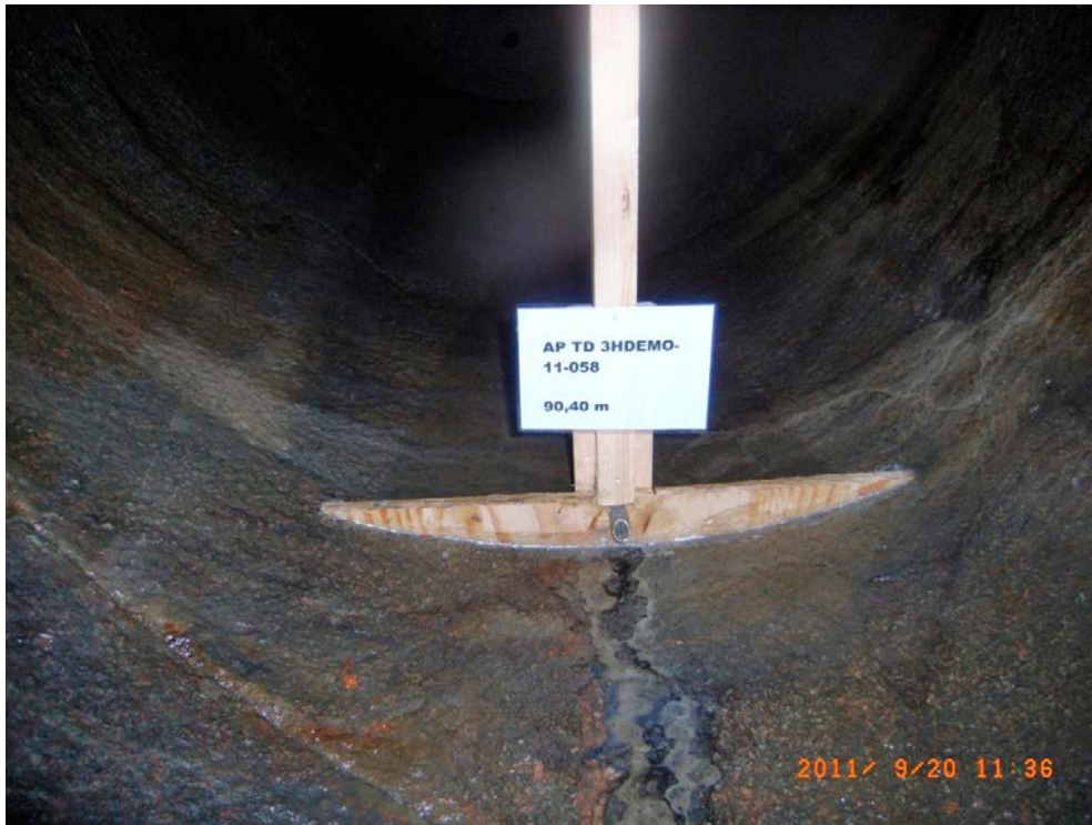
Figure 3-1. Wooden weir used to section off and measure the distribution of groundwater inflow in the MPT section.
