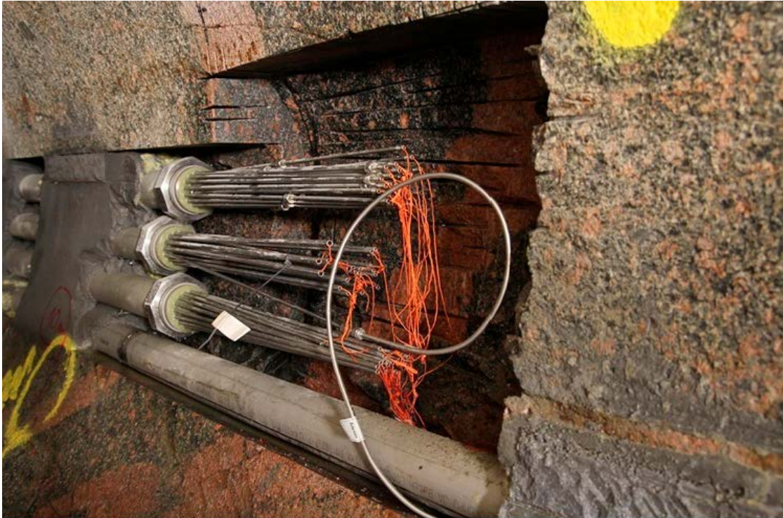
Figure 5-9. 'Hedgehog' connectors at the Supercontainer position, in this case three 'hedgehogs' due to the numerous sensors inside the Supercontainer. The pipe passing by at the bottom carries the sensor cables from the innermost distance block. The small pipe in a loop and already connected is from one of the rock-sensors.
