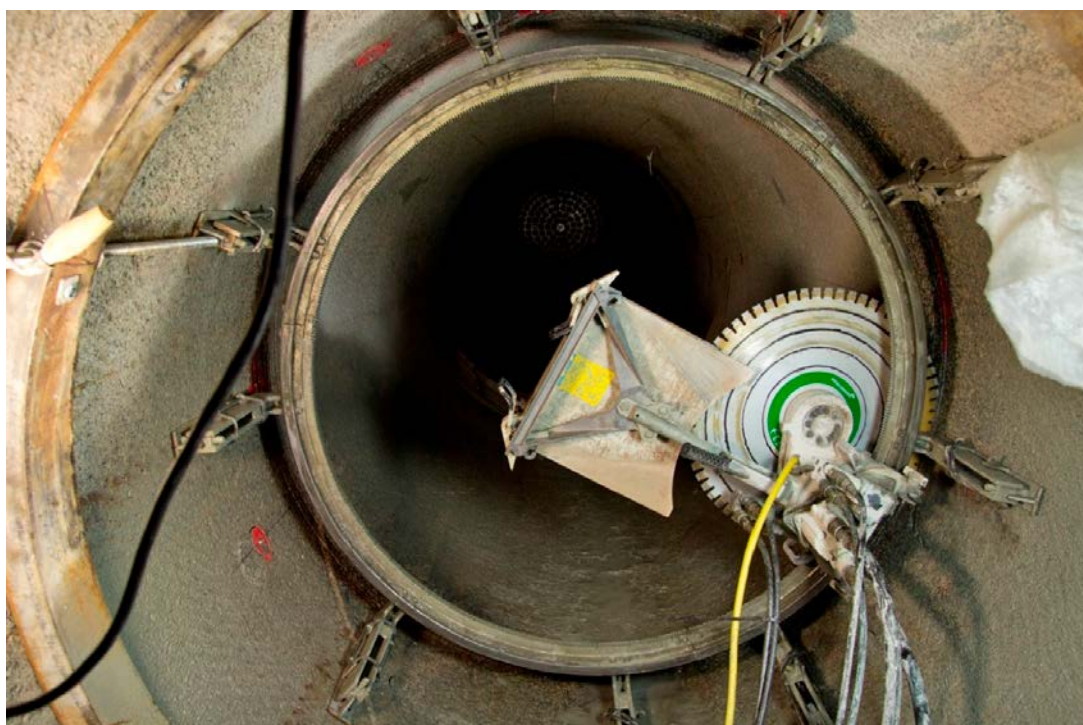
Figure 5-1. Rail and saw installed inside the drift. The reference ring towards which the rail is pulled in 45 mm steps can be seen to the left in the picture.
