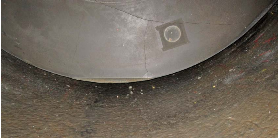
Figure 9-5. Crack on the inner distance block which was noted when the cable block was removed.
