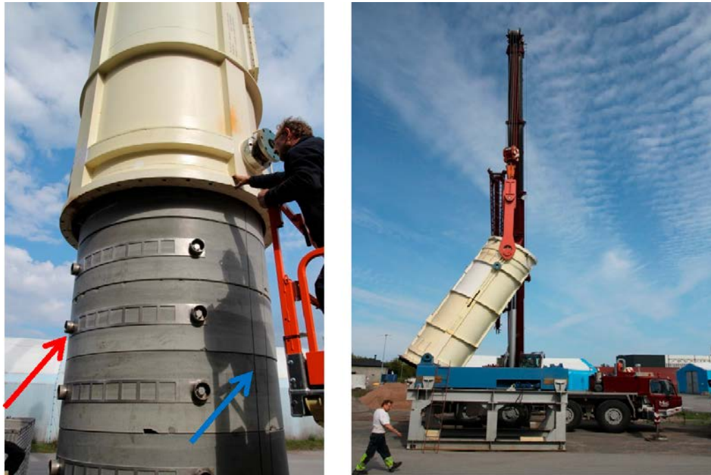
Figure 7-4. The transport tube is being lowered over the distance block (left). The feet placed on each distance block segment are clearly visible (red arrow) and two cable pipes milled into the block surface can be seen to the right of the component (blue arrow). The transport tube is being lowered on to its transport cradle (right).
