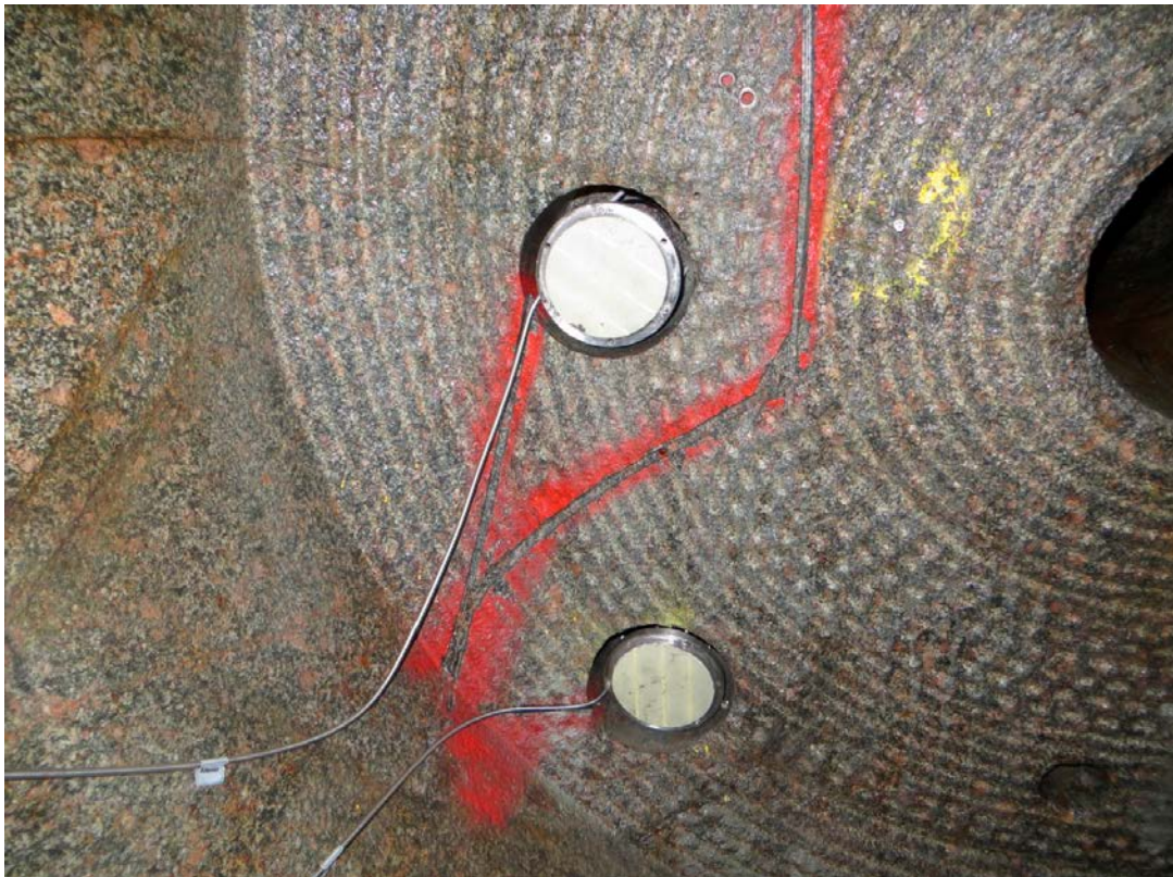
Figure 5-7. Total pressure sensor position in their holes prior to casting. The picture, which is taken at the drift end, also illustrates the shallow cutouts in which the sensor cable pipes were placed (red spray on the wall).
