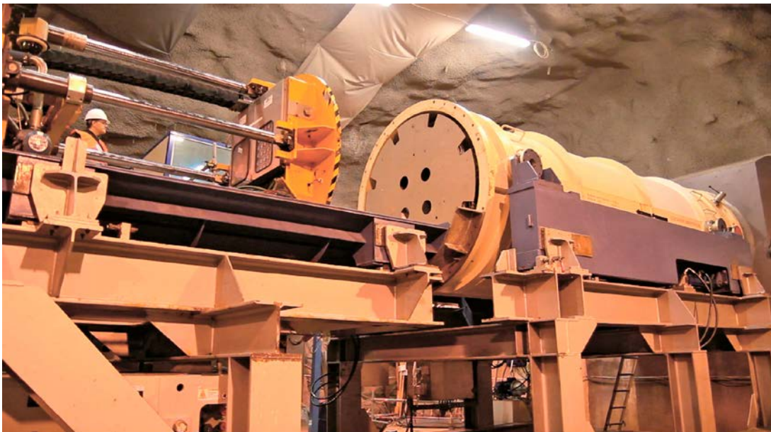
Figure 7-7. Starting- and transport tube aligned in front of the drift, being ready for deposition. The test distance block is inside the transport tube with only the bottom of the cable block visible.
