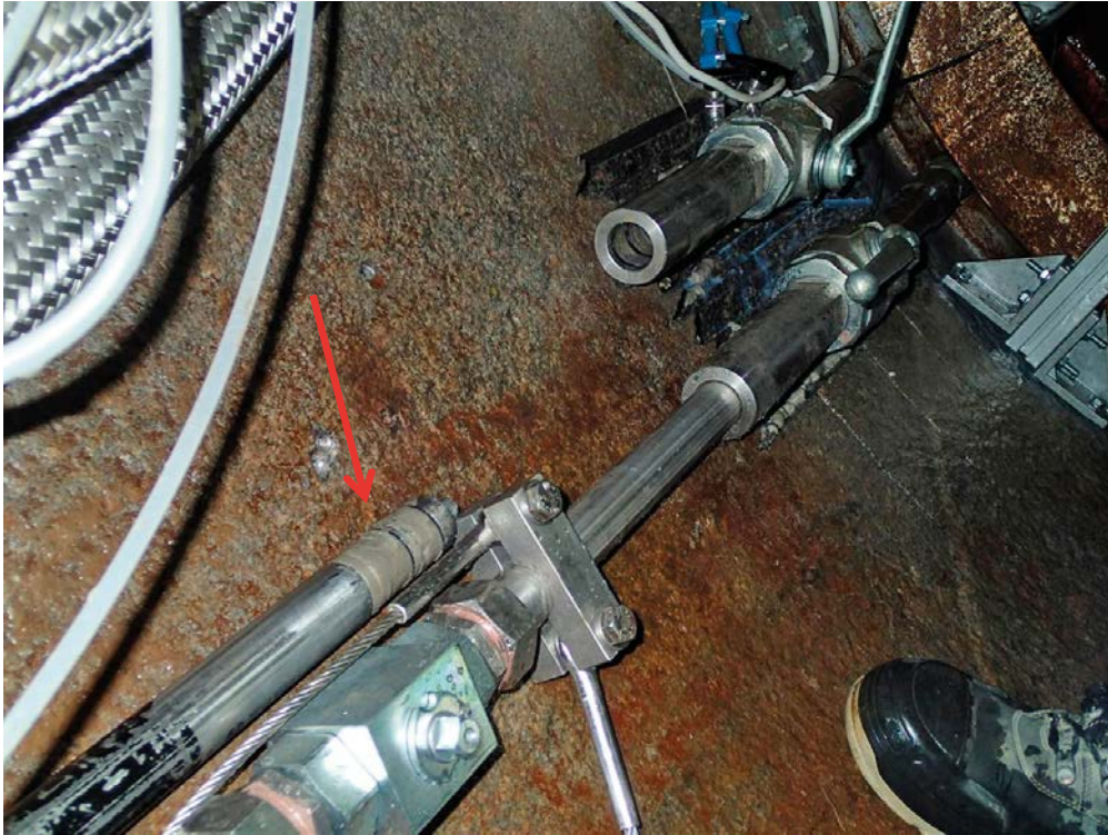
Figure 9-20. The air evacuation pipe has just been pulled out and the first water filling pipe is connected with a wire to be pulled out. Bentonite can be seen stuck to the valve part of the air evacuation pipe (red arrow).
