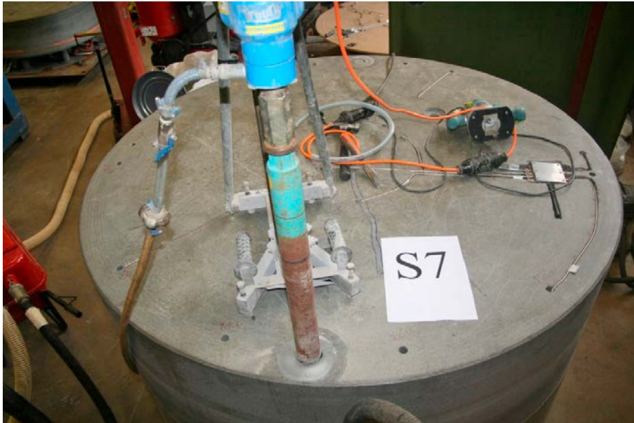
Figure 8-2. Drilling for placing sensors in section 7, one of the wireless transmitters and its sensors has already been placed, to the right.
