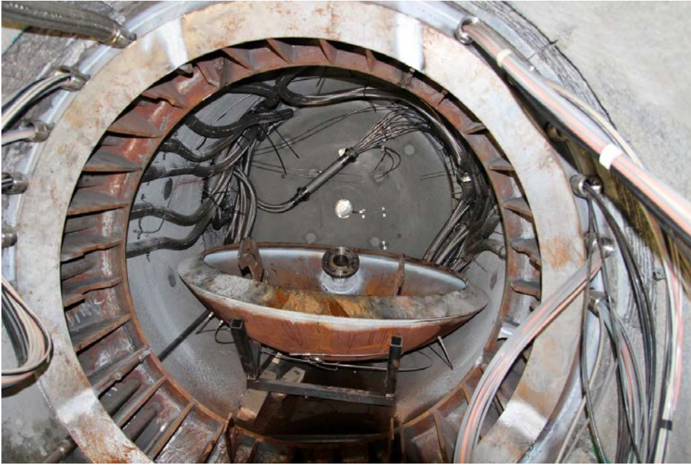
Figure 9-11. The flexible pipes between the collar and the main wall pipes can be seen attached on the drift wall between the collar and the transition block.
