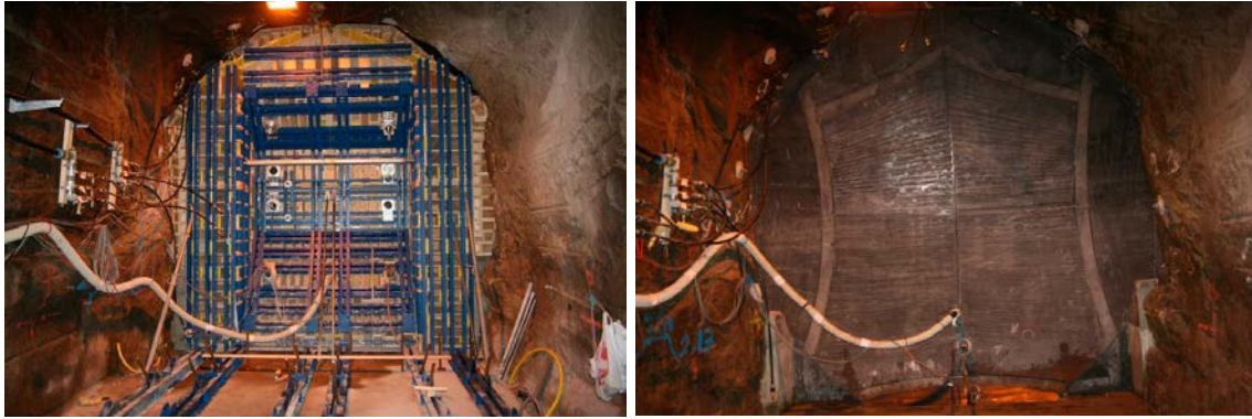
Figure 3-4. View of the form without the stiffeners before casting (left) and of the concrete dome plug after removal of the form (right).
