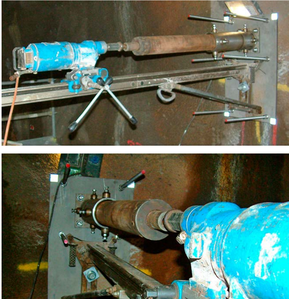
Figure 4-9. Aligning equipment developed by the KBS-3H project for drilling casing holes with high accuracy.
