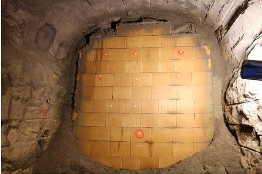
Figure 4-28. The full-scale backfill installation is completed at Äspö HRL. 84.5 tons of pellets and 380 tons of blocks were installed in 12 m of tunnel.
