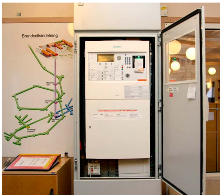
Figure 6-3. Control panel for the new fire alarm system in the Äspö HRL.
