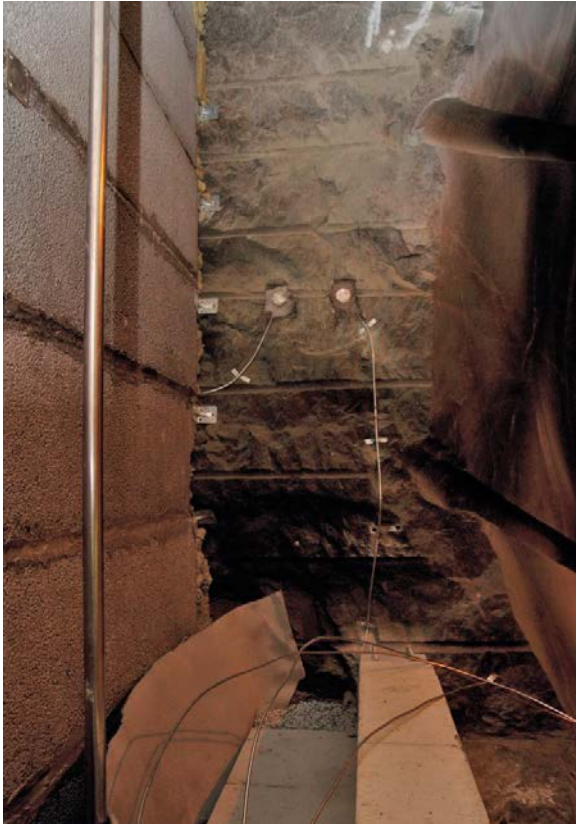
Figure 4-31. Detail photo showing (from left) filter of leca-beams and macadam, drainage (air) pipe, geotextile, bentonite seal of MX-80 (blocks and pellets) and concrete delimiters. All sensor cables are led in steel tubes.
