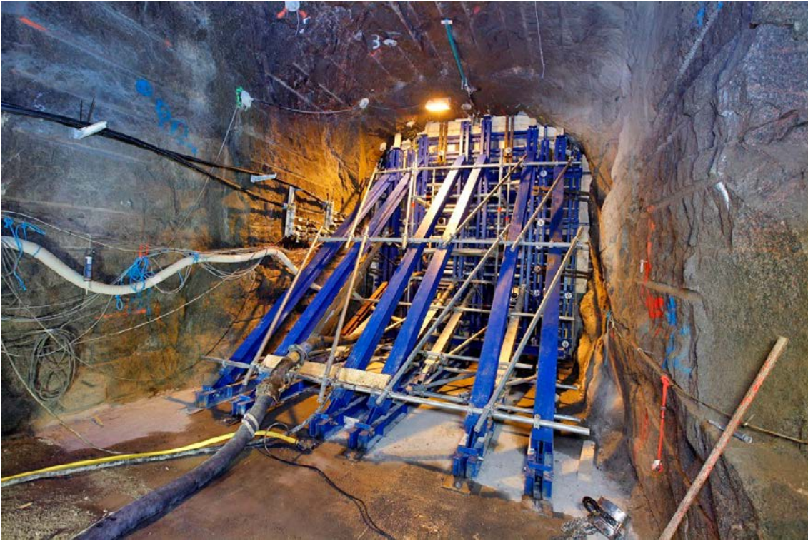
Figure 4-33. Concrete is pumped in behind the formwork for casting of the concrete dome structure.
