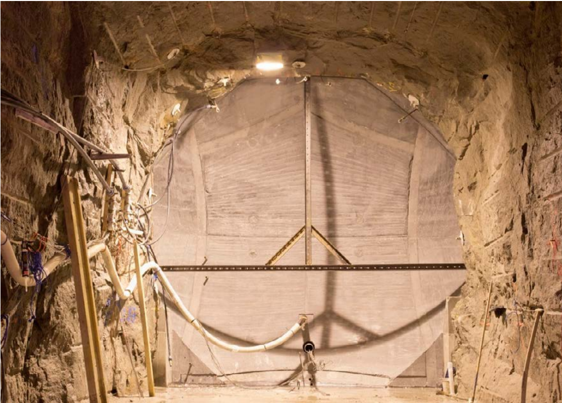
Figure 4-34. The hardened concrete dome structure after removal of formwork. The steel beams in front of the dome are used for displacement sensors.
