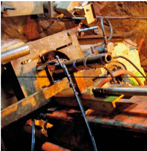
Figure 3-13. The sledge holding the tool for breaking, lined up to be connected to the drill stem for lowering into the hole.
