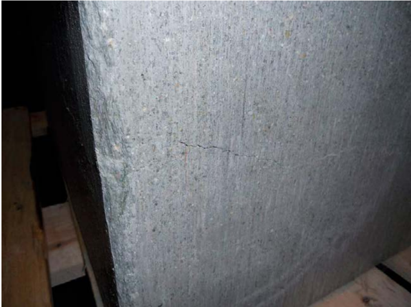
Figure 5-6. Close-up photo showing one of the first blocks made of IBECO. The photo shows the fragile edges and a part of a horizontal crack.
