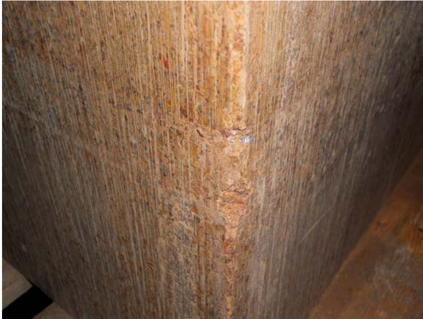
Figure 5-5. Close up showing one of the block edges. All edges were very fragile and material loosened easy from the block.
