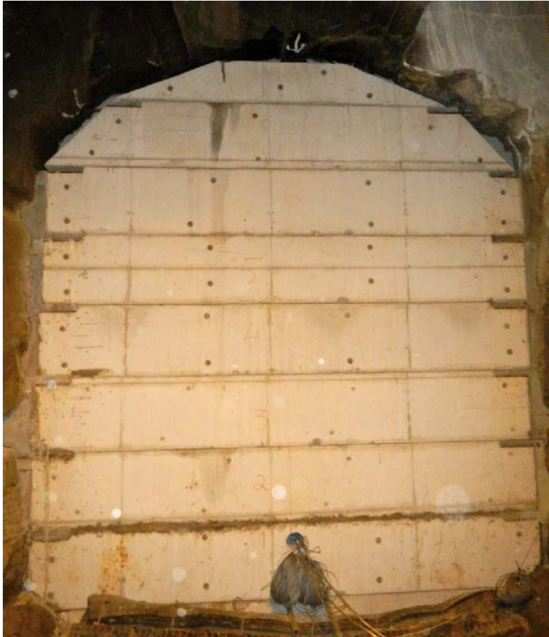
Figure 6-3. Photo showing an example of a temporary plug. The concrete beams are of the same type as the one suggested for a plug of class III and IV. The photo was taken during the installation of the Dome Plug project at Äspö HRL (Report in prep.).
