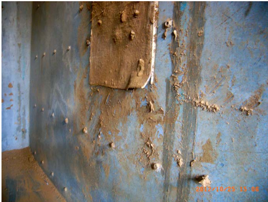
Figure 4-15. Photo of the loosened geotextile.
