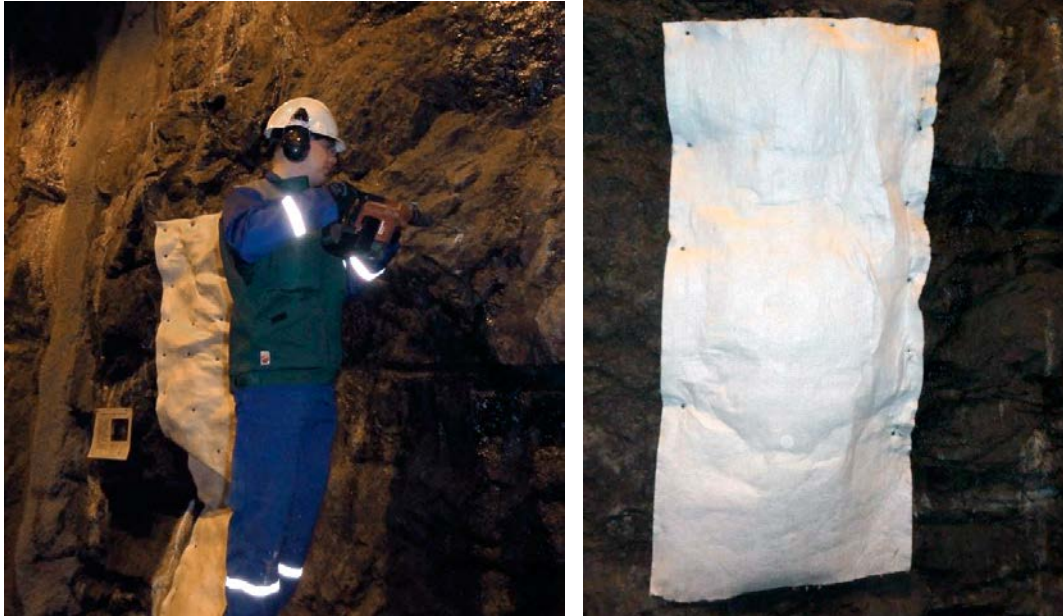
Figure 5-3. On the left, the fastening process and on the right the glass fibre fabric installed on the rock wall.
