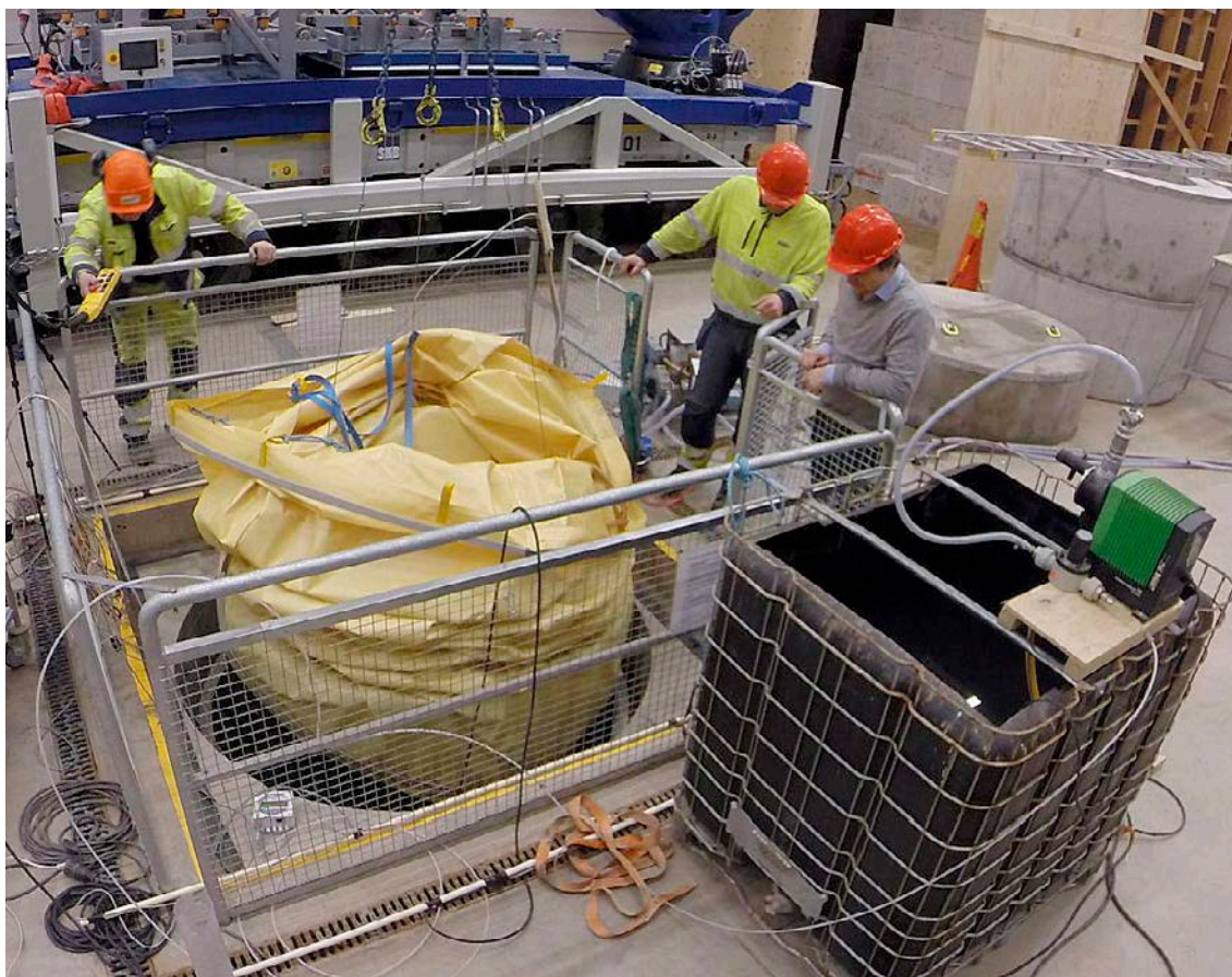
Figure 4-2. Photo taken when the assembled bottom plate and buffer protection sheet were lowered into the deposition hole in the bentonite laboratory at Äspö.
