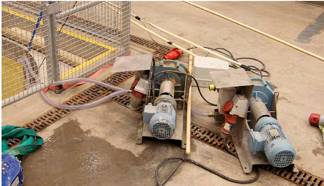
Figure 3-6. Water evacuation equipment.
