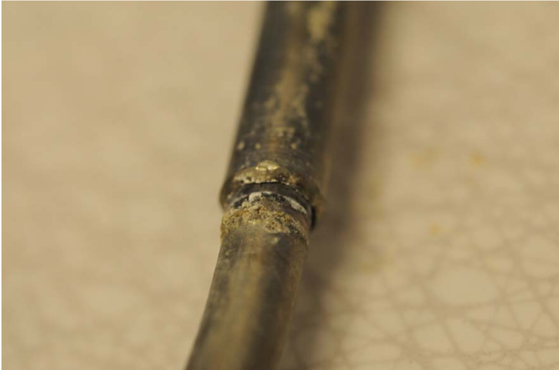
Figure B-9. Sensor Geokon 70064, weld 8 mm to 6 mm tube has broken and water can reach the sensors electronics.
