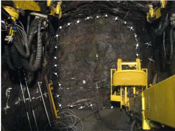
Figure 4-21. Although the repository facility will be located in rock mass of good quality with most relatively low fracturing, sealing by means of rock grouting will be necessary.
