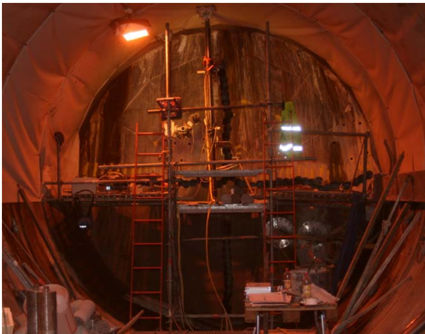
Figure 4-5. Breaching of the outer plug in December 2010 with the core drilled holes before hydraulic splitting.
