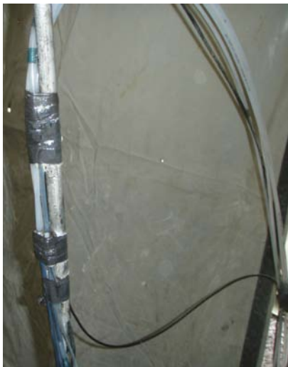
Figure 3-9. Parts of the instrumentation in a core drilled borehole. Pipe string and tubing attached with black tape. The instrumentation in core drilled boreholes is used for pressure measurements and chemical monitoring.
