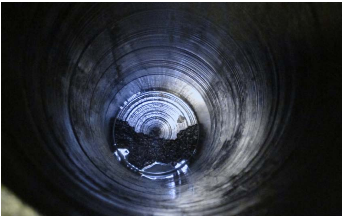
Figure 3-13. One of two central boreholes (300 mm) in TASO-tunnel for installation of bentonite.
