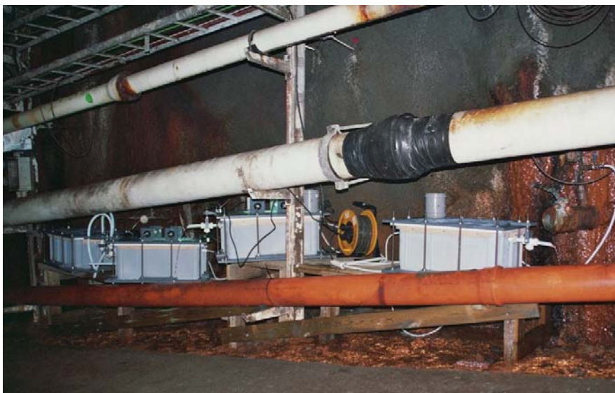
Figure 7-6. Flow reactor set (white boxes) installed at TASA 1327B.
