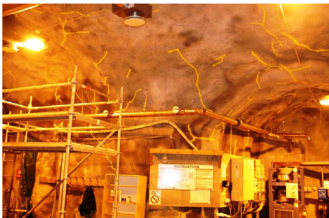
Figure 2-3. TASL-tunnel. Irregular fractures marked with yellow paint in the ceiling and on the walls.
