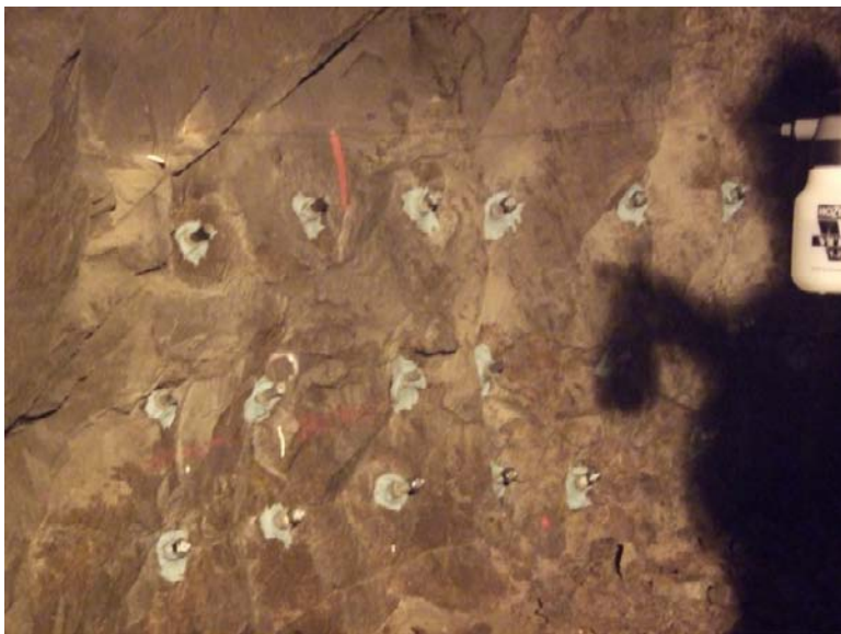
Figure 7-12. Mounted rock bolts in the Äspö tunnel are sprayed once a month during one year.
