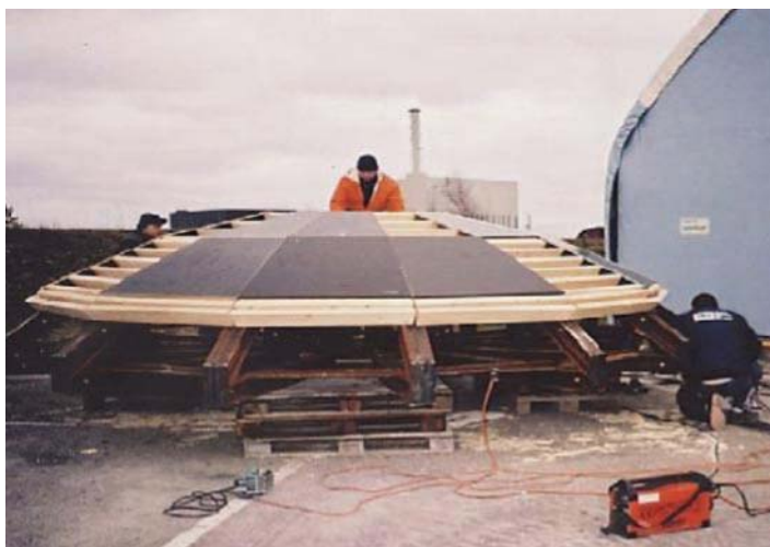
Figure 2-8. Formwork for the downstream side of the dome shaped concrete plug, used in the Prototype Repository.
