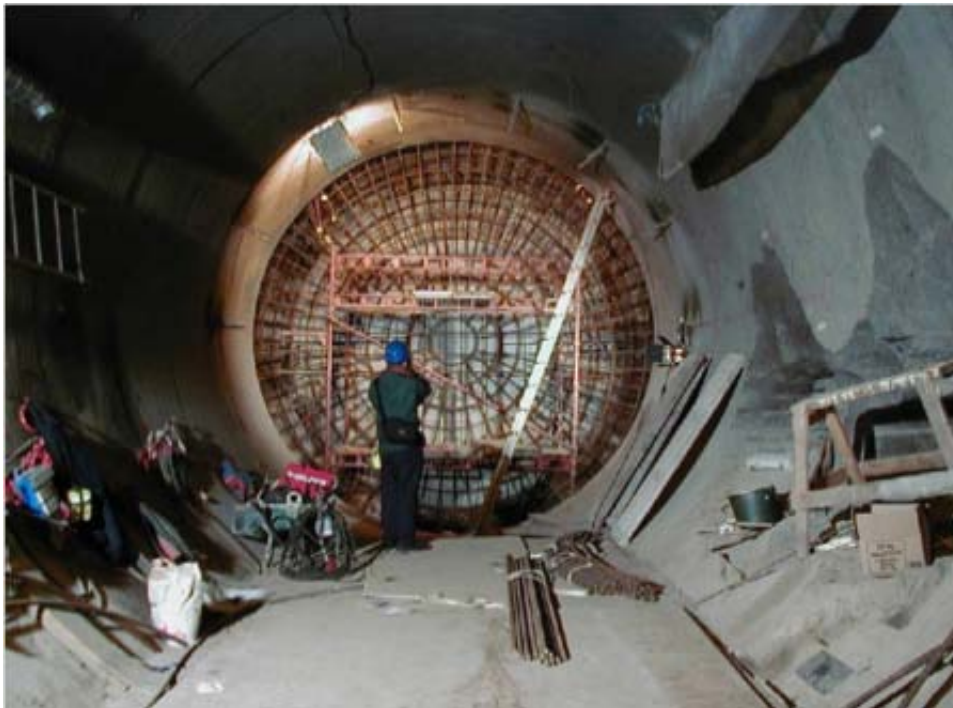
Figure 1-10. A photo of the reinforcement in Plug II in the Prototype Repository.
