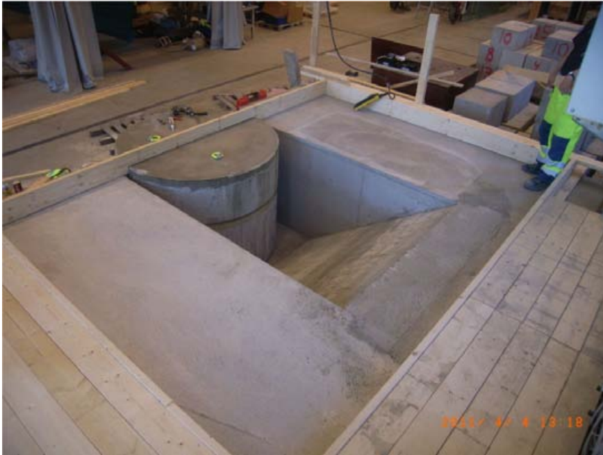
Figure 2-14. The upper part of a deposition hole with buffer block and bevel was modelled with concrete in full scale.
