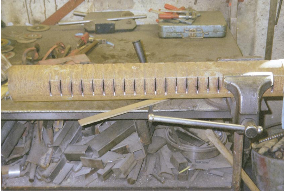
Figure 4-3. Drill casing used as a combined screen and pipe in pumping well SFM0074 under construction at SWECO's engineering workshop in Stockholm. The custom-made screen is perforated by openings with a length of 40 mm and a width of 3 mm.
