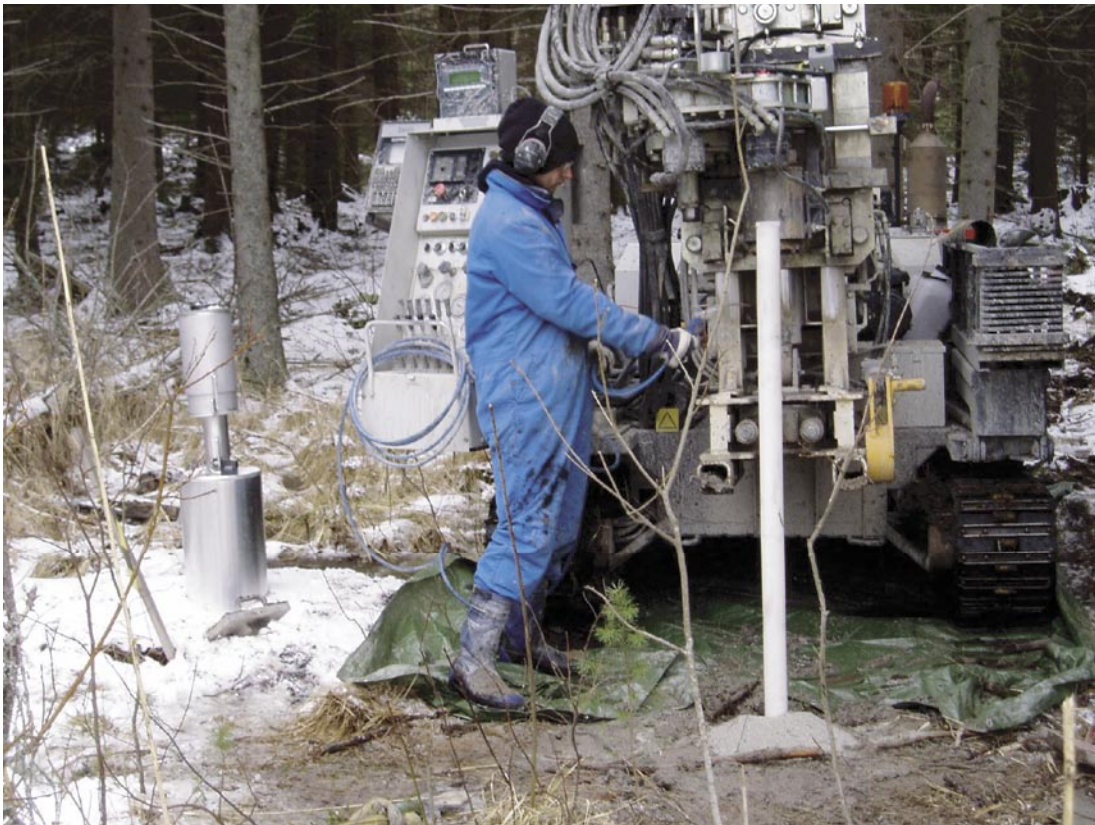
Figure 3-1. Installation of groundwater monitoring well SFM0068. A GeoMachine GM 100 GTT drilling rig with a 8-bars Dynaset air compressor was used for installation of all groundwater monitoring wells in soil.
