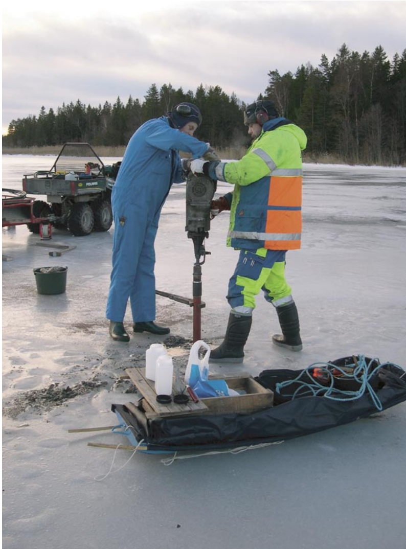
Figure 3-2. Installation of groundwater monitoring well SFM0022. A hand-held Berema Pionjär was used for installation of all groundwater monitoring wells below open water and surface water level gauges.
