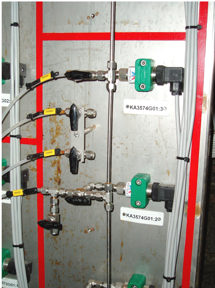
Figure 4-2 Pressure transducers connections
