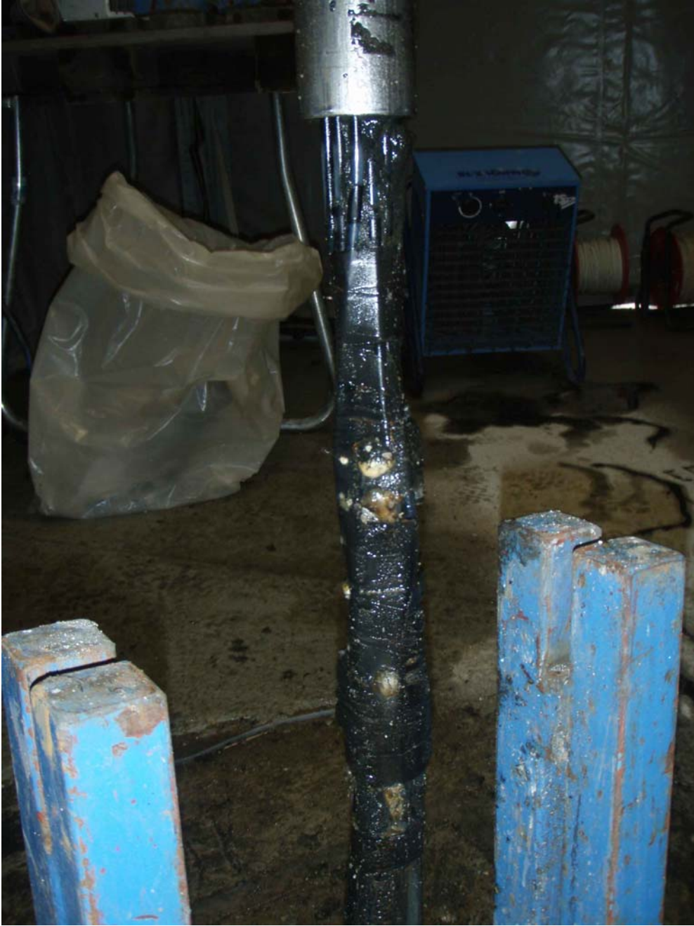
Figure A5-3. Bottom of standpipe (stainless steel) in KAS03. Tubing for pressure measurements and water sampling hold together by black tape (PVC).
