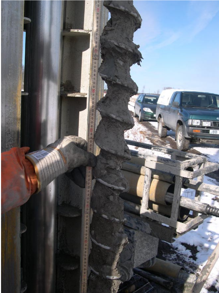
Figure 3-3. Clayey till retrieved by auger drilling at the installation of groundwater monitoring wells /Johansson, 2003/. The till stratigraphy was investigated by /Hedenström et al, 2004/.
