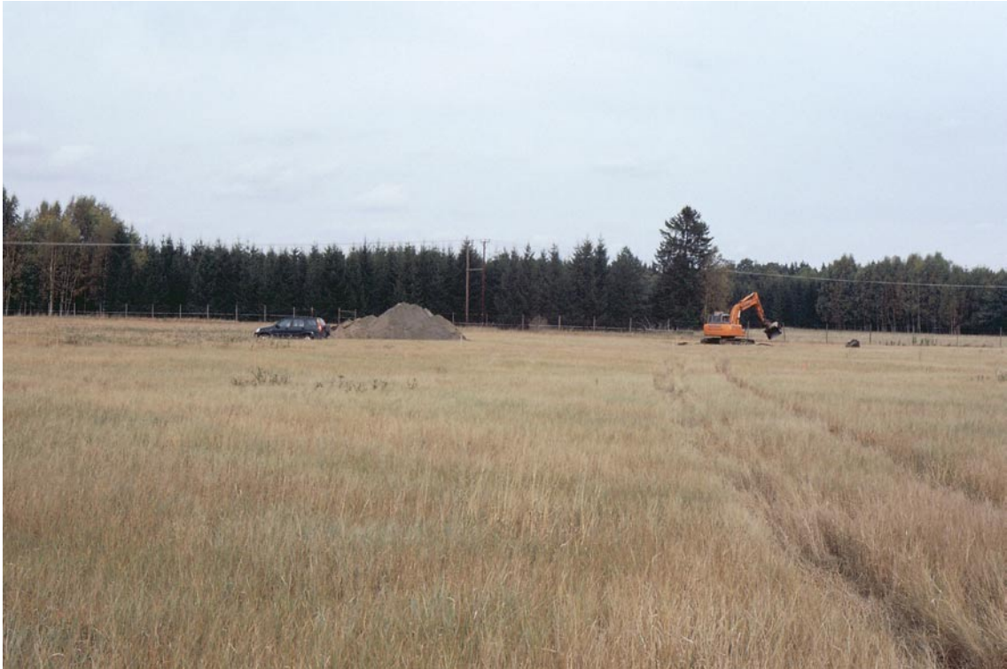
Figure 4-2. Typical excavation site in very gently sloping ground along the Börstil esker. Kråkmötet (E4) after opening of a first test pit.
