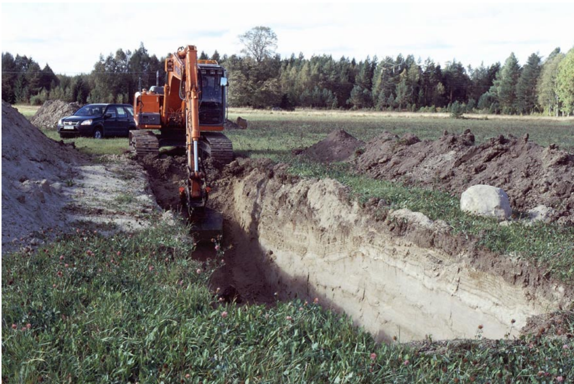
Figure 3-1. During 2003 the activities within the project were focussed on stratigraphical investigations in machine-cut trenches. Crawler excavators capable of cutting trenches to a depth of some 5 metres were used. Trenching at Hultet, E3 in Figure 4-1.
