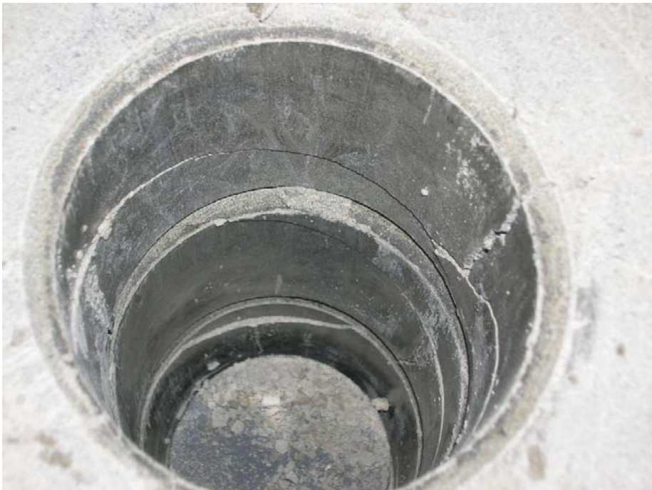
Figure A2-4. Photo taken during excavation. The large cracks in the blocks are very clear.
