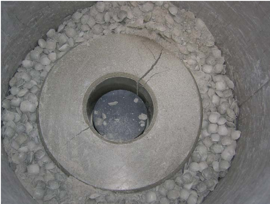
Figure A9-4. Picture showing the bottom block. Only a small part of the pellets are affected of the water. The block has cracked diametrically.
