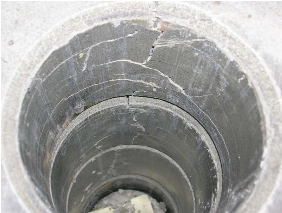
Figure A7-4. Photo taken during excavation. The large cracks in the blocks are very clear.
