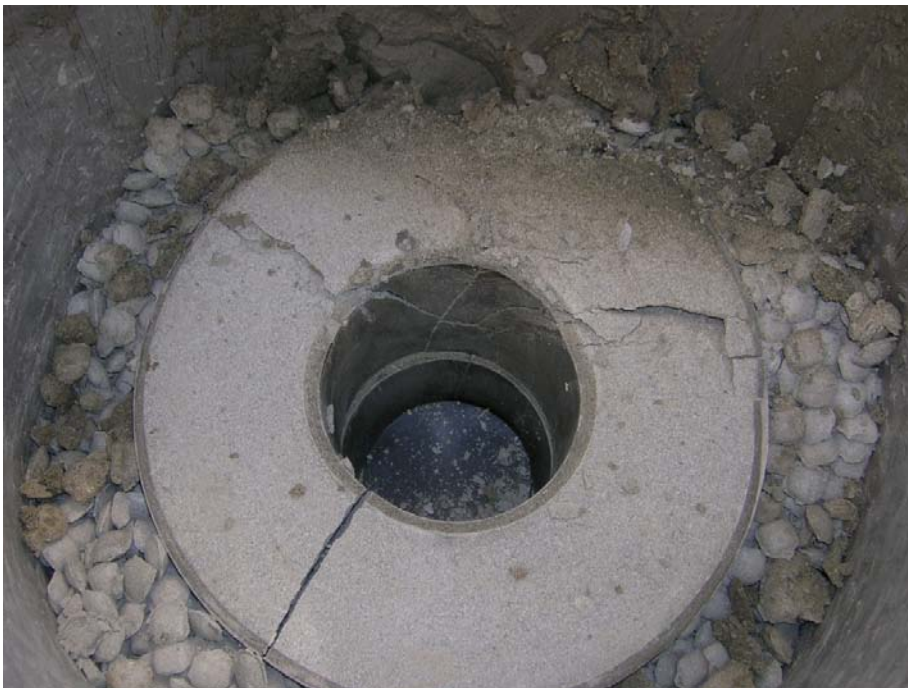
Figure A6-4. Photo taken during excavation. The large cracks in the blocks are very clear. Only parts of the pellet filling is wetted.
