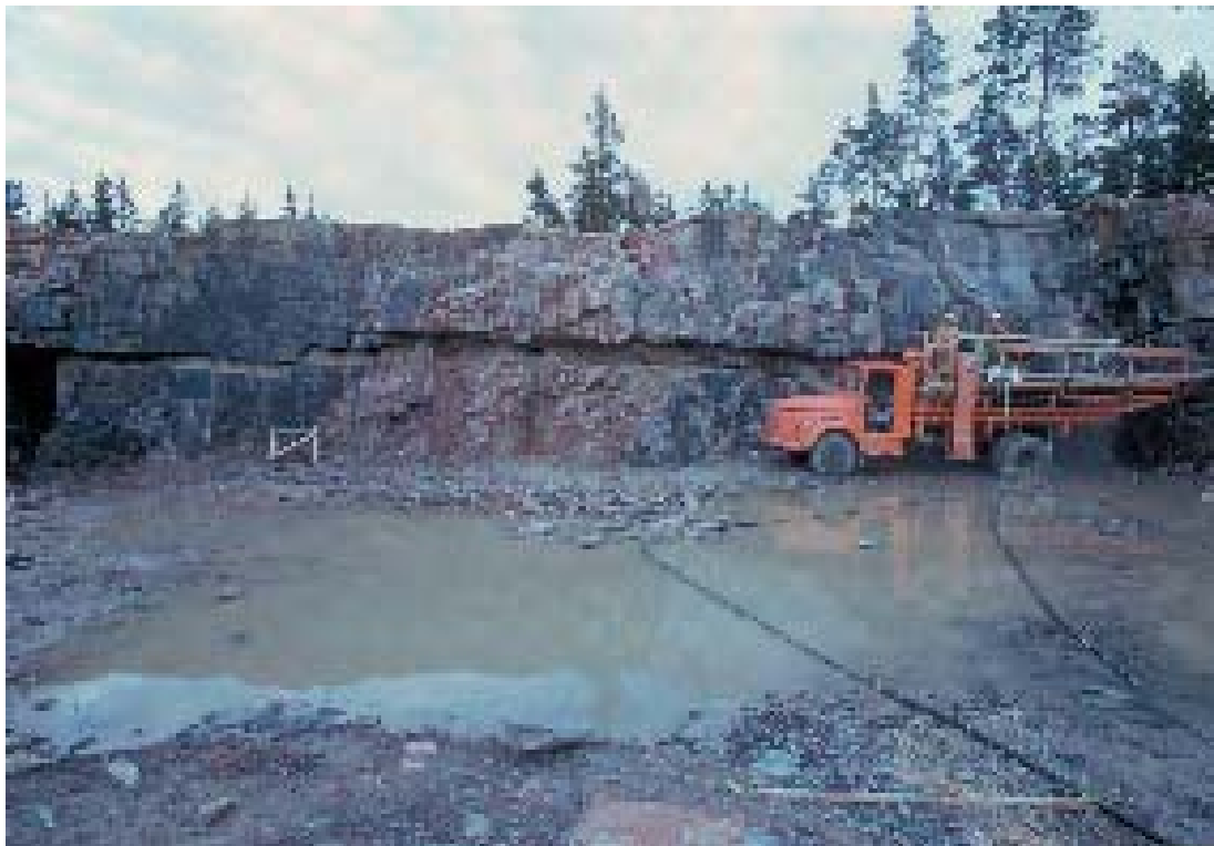
Figure 4-60. View of excavations of Unit #3. Notice the sediment-filled horizontal fracture /Carlsson, 1979/. The rock mass is rather blocky with some more fractured zones. Generally, the fracture frequency at surface decreases within the depth of the excavations.
