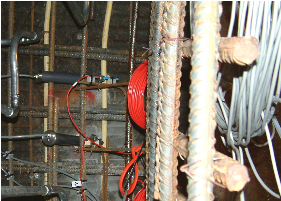
Figure 6-3. Installed instruments for monitoring the mechanical response.
