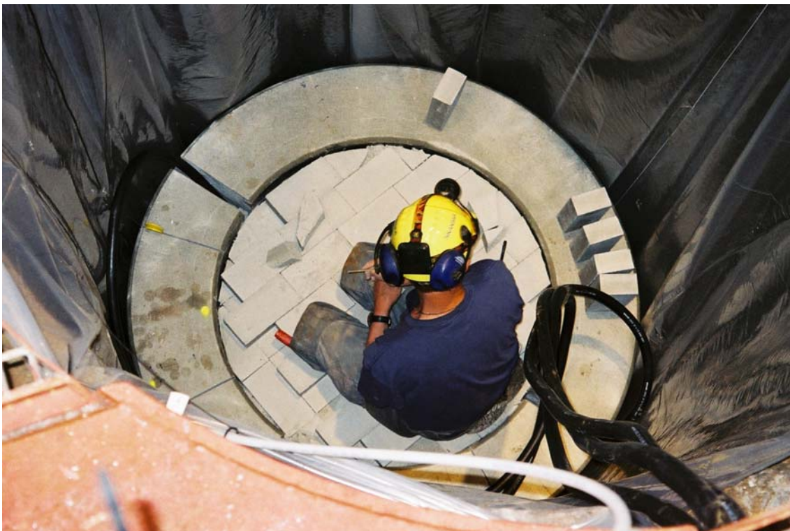
Figure 4-8. Bricks of bentonite placed on top of the lid of the canister.
