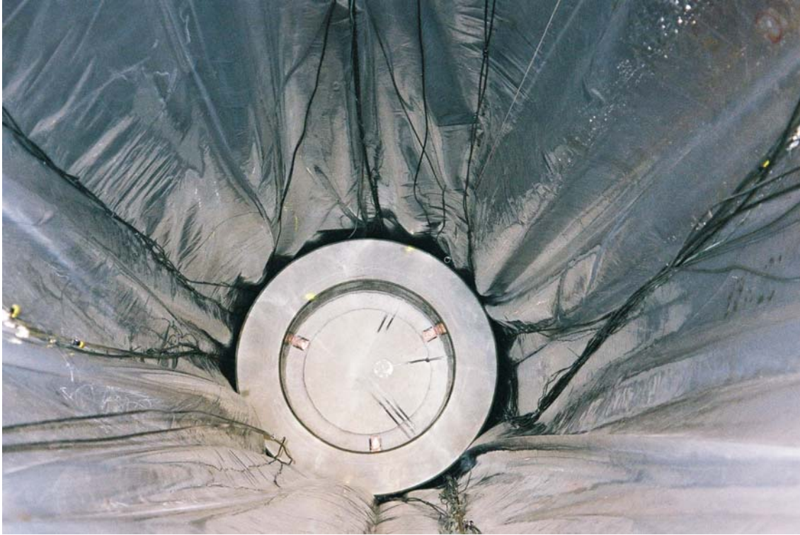
Figure 4-3. A photo taken after installation of the bottom block and the first bentonite ring, showing also the plastic sheet and several transducers installed in the bottom block.
