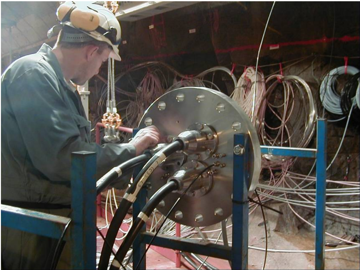
Figure 2-6. Photo showing the assembling of a cable parcel with cables from canisters.
