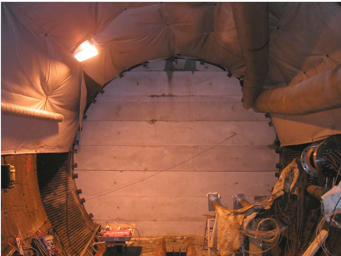
Figure 5-15. All nine concrete beams and the two lead through pipes in place.
