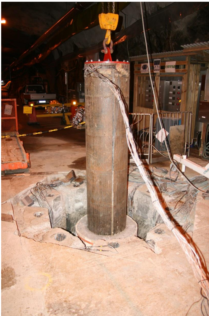
Figure 4-1 The lifting of the lower heater in the excavation of the Temperature Buffer Test.
