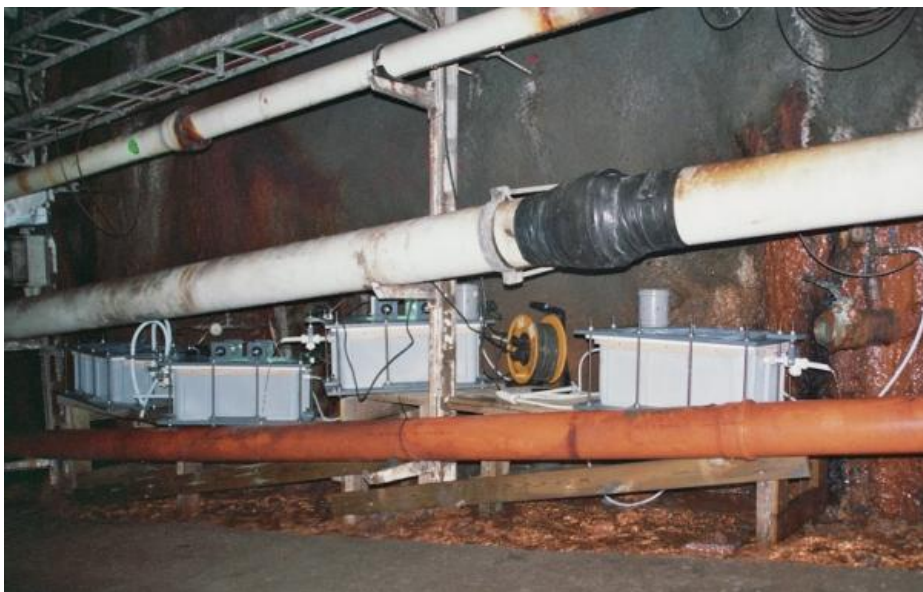
Figure 7-6. Flow reactor set (white boxes) installed in the Tasa-tunnel in 2006.
