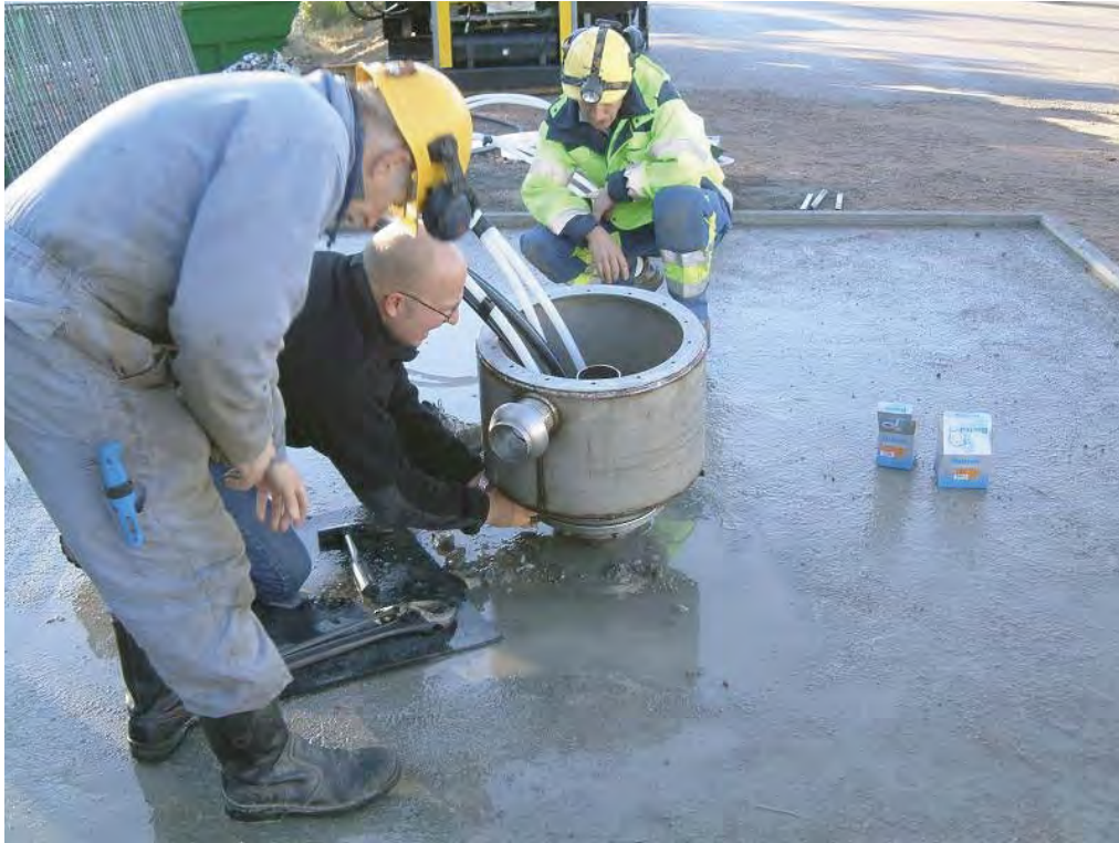
Figure 5-8. Fitting the flushing water discharge header. The supportive casing and the hoses for air-lift pumping can also be seen.
