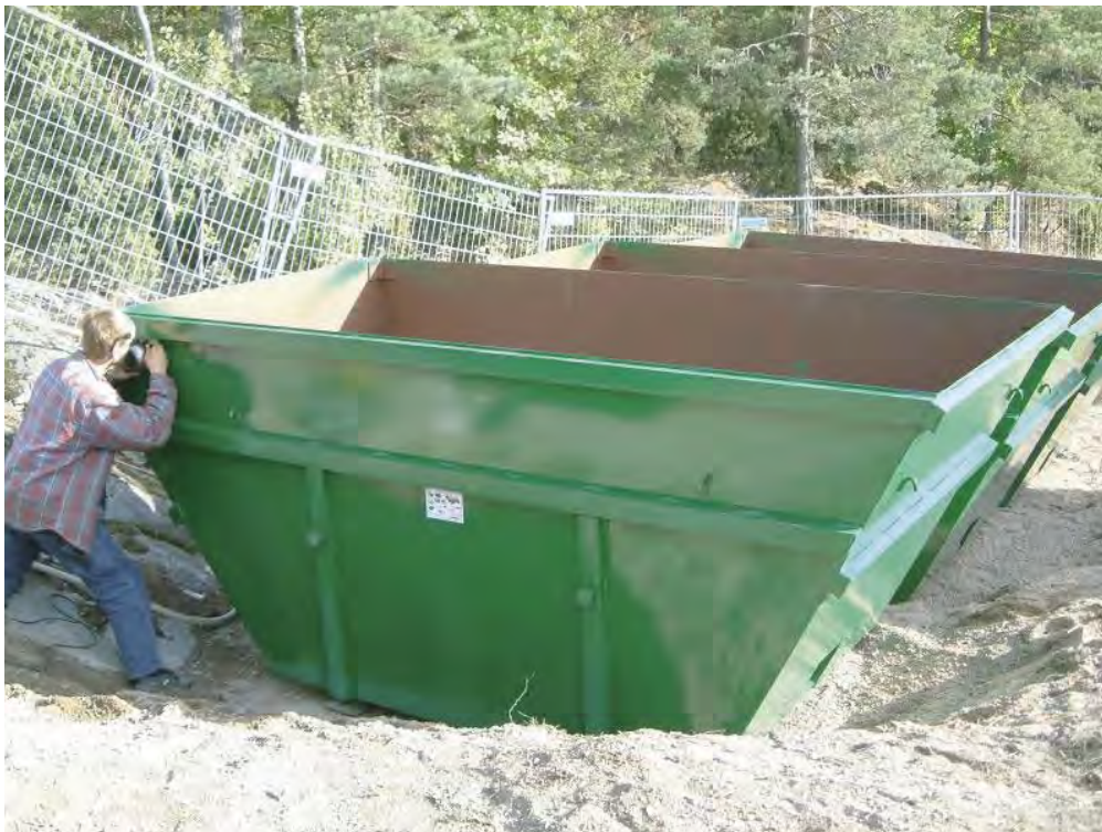
Figure 5-9. Aligning the flushing water discharge containers. The sludge and cuttings is allowed to settle in the containers.
