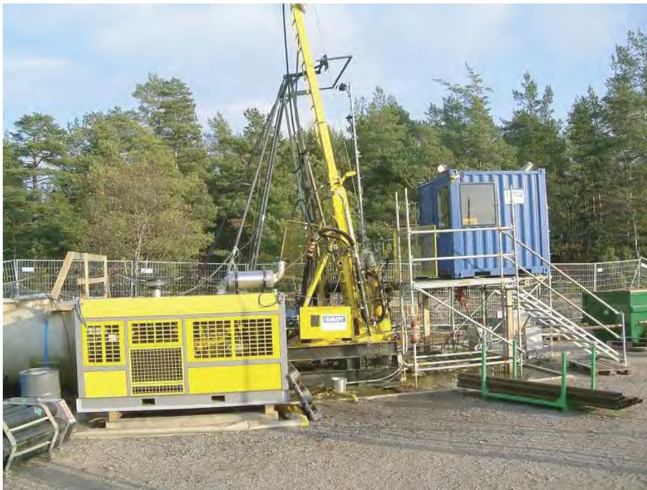
Figure 4-1. Compressor and drill rig. Gas tubes for nitrogen saturation and the flushing water tank can be seen in the lower left corner.
