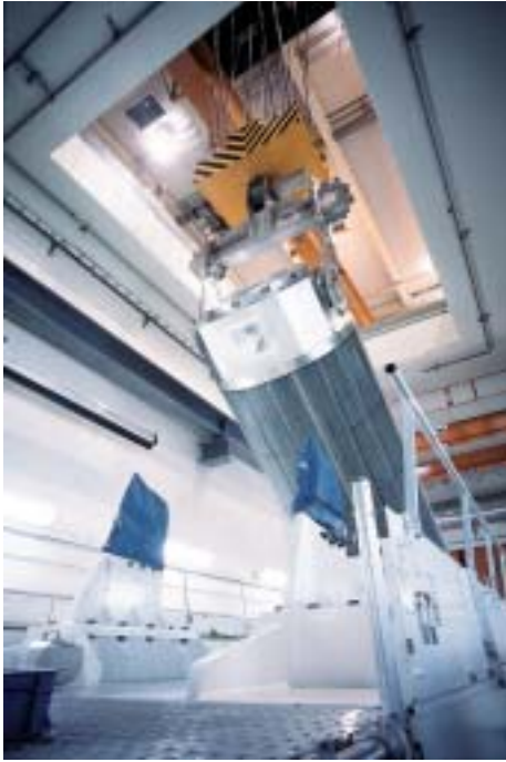
Handling of transport cask in the receiving section.
