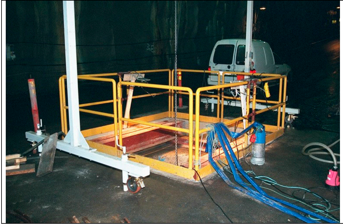
Appendix 11A. Photos from deposition hole DA3147G01 (photos: Lars Andersson, SKB). Top of the hole with safety fence and part of the lift.
