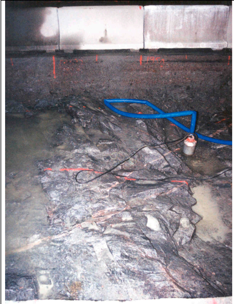
Appendix 8C. Photos showing the pit-floor in the TBM assembly hall (photos: Lars Andersson, SKB). Section 3/148-3/153, Äspö diorite (grey) with fine-grained granite veins (pinkish red)
