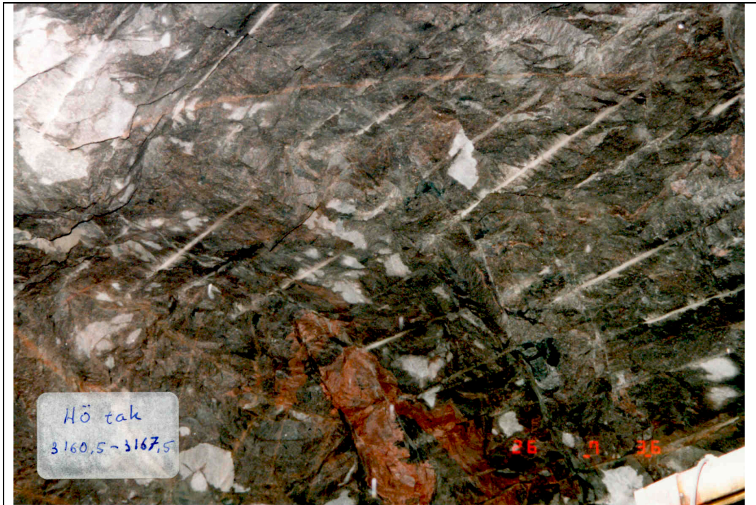
Appendix 3C. Photos showing the interior of the TBM assembly hall (photos: Geologist team at the time, SKB). Roof, right side, section 3/160.5-3/167.5. Mainly Äspö diorite (grey) with some fine-grained granite (brownish red).
