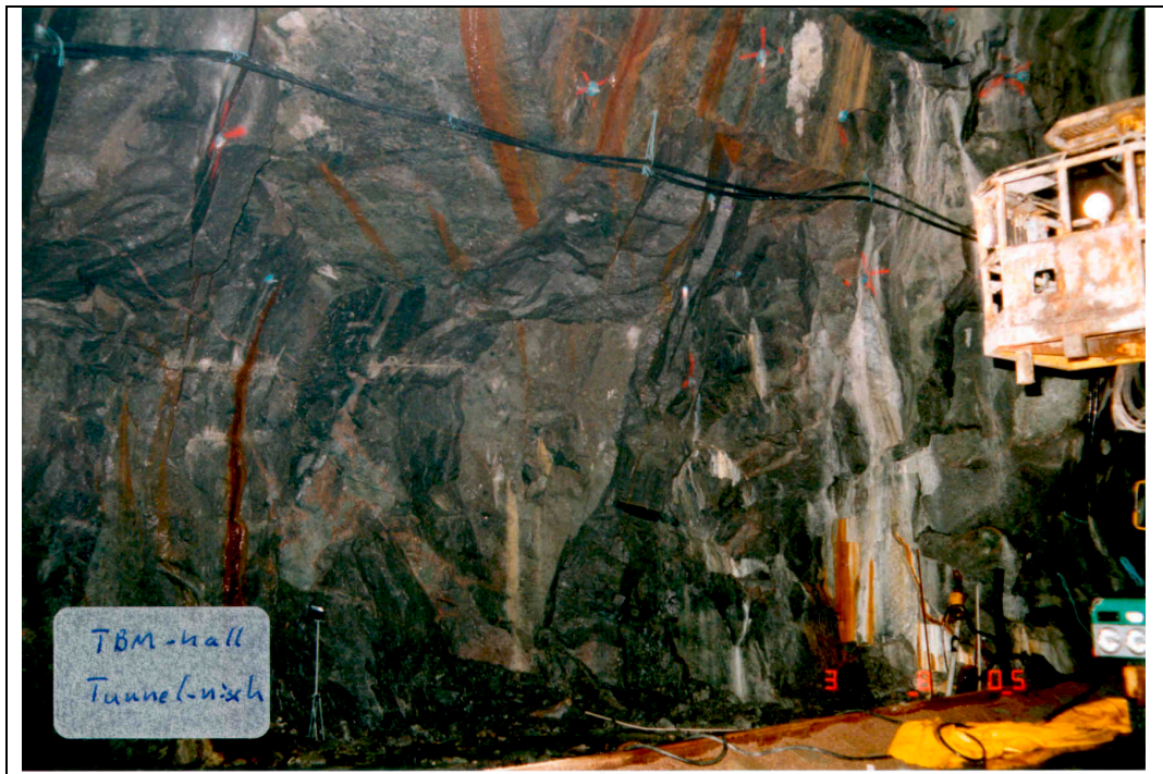
Appendix 3A. Photos showing the interior of the TBM assembly hall (photos: Geologist team at the time, SKB). Small niche, left side wall. Mainly Åspö diorite (grey).
