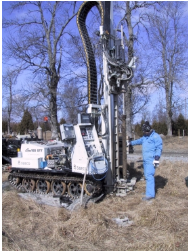
Figure 3-1. Drilling rig GeoMachine GM 100 GTT with a 8 bar Dynaset air compressor was used for most of the work.
