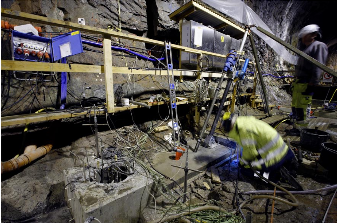
Figure V-15. Shows the core drilling of the water injection holes used in the post characterization damage zone in KQ0046G03.
