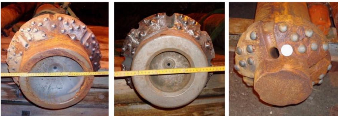
Figure 4-2. A photograph of the equipment used for reaming the heating holes with close-up views of some of the drill bits that were utilized (Photo R Glamheden).
