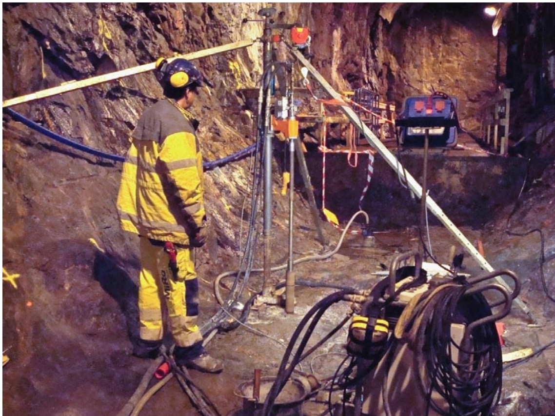
Figure 4-1. A photograph of the equipment used for the core drilling (Photo R Glamheden).
