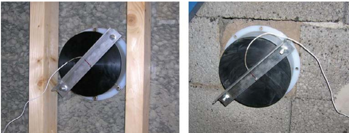
Figure F-7. Left: Pressure cell mounted on the “bentonite” side. Right: Pressure cell mounted on the “rock” wall.
