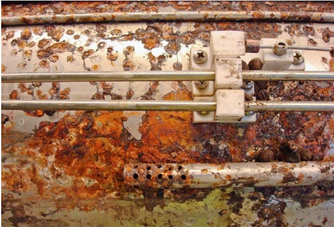
Figure 5-2. Illustrates the corrosive degradation process the test equipment was exposed to during the heating tests. The photograph shows part of the large tube and the minor tube for the upper RH-gauge from hole KQ0048G04 in Test 3 (Photo R Glamheden).
