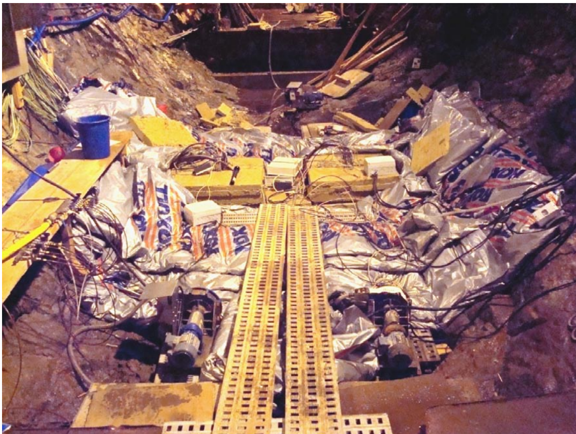
Figure 4-7. The test site just before starting the second field test (Photo R Glamheden).
