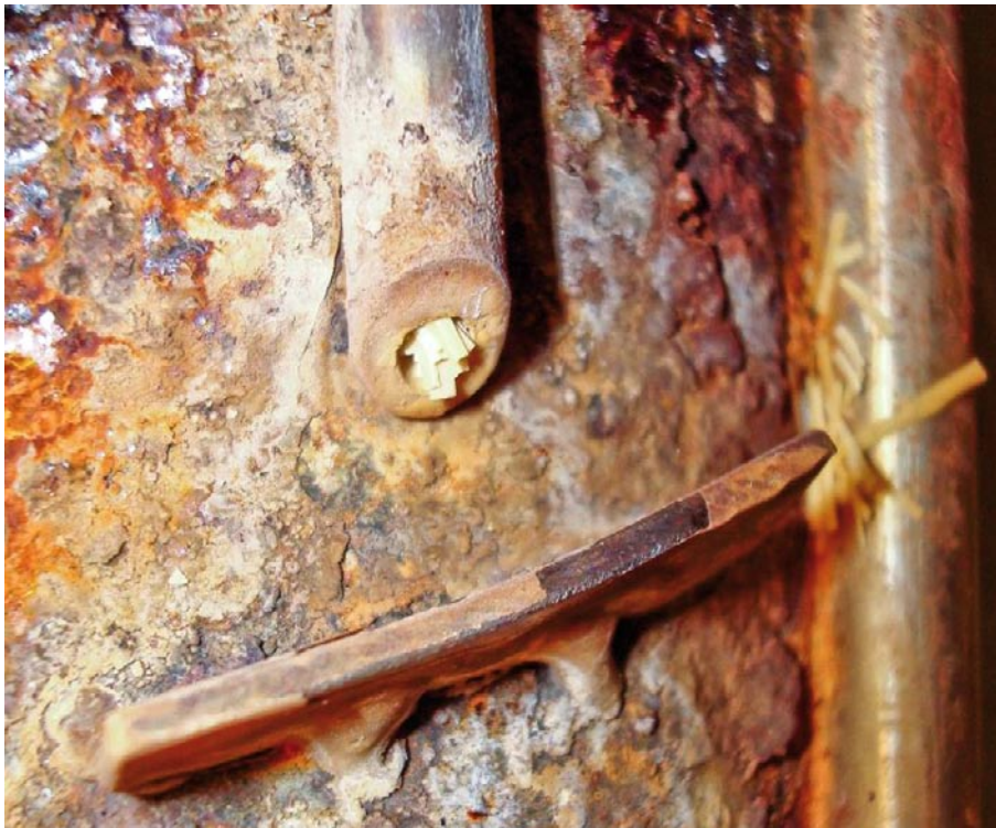
Figure U-9. Shows a close-up view of one of the drip holes in the wetting system after completion of Field Test 2.
