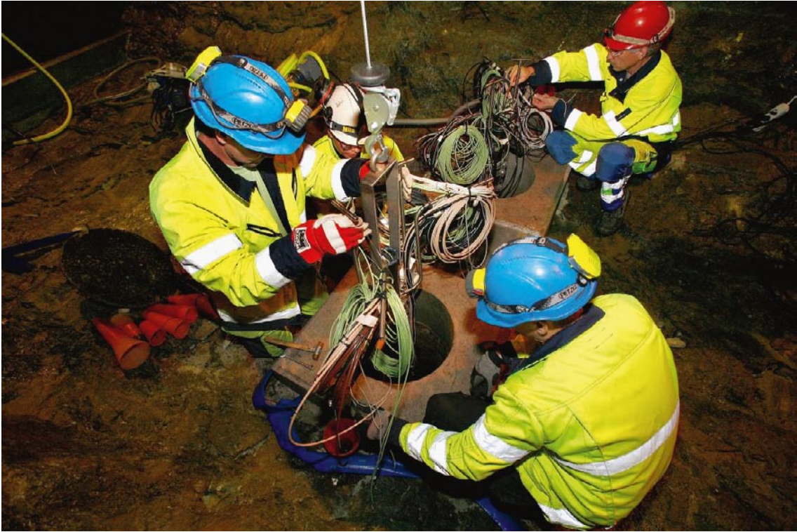
Figure V-2. Shows the test equipment in place in Field Test 1.
