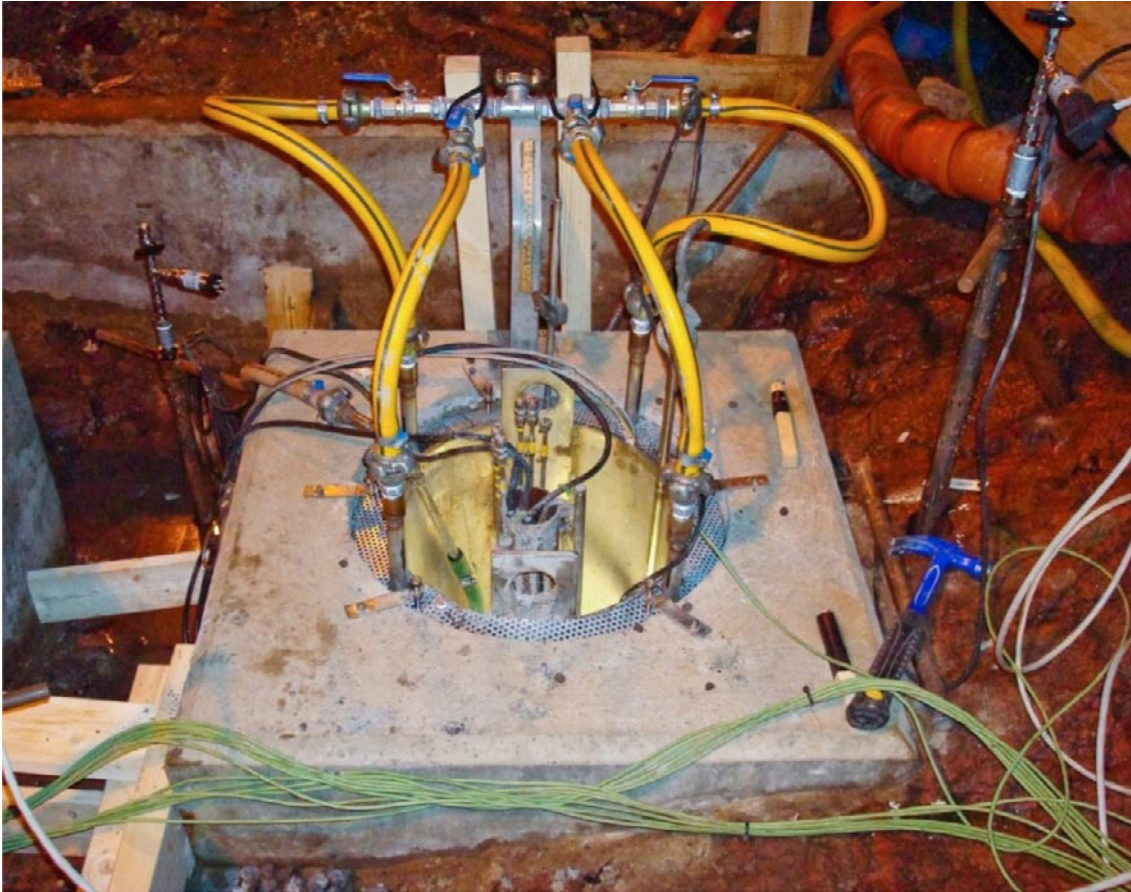
Figure 7-9. A top view of the pellet filled slot before the start of grouting (Photo R Glamheden).
