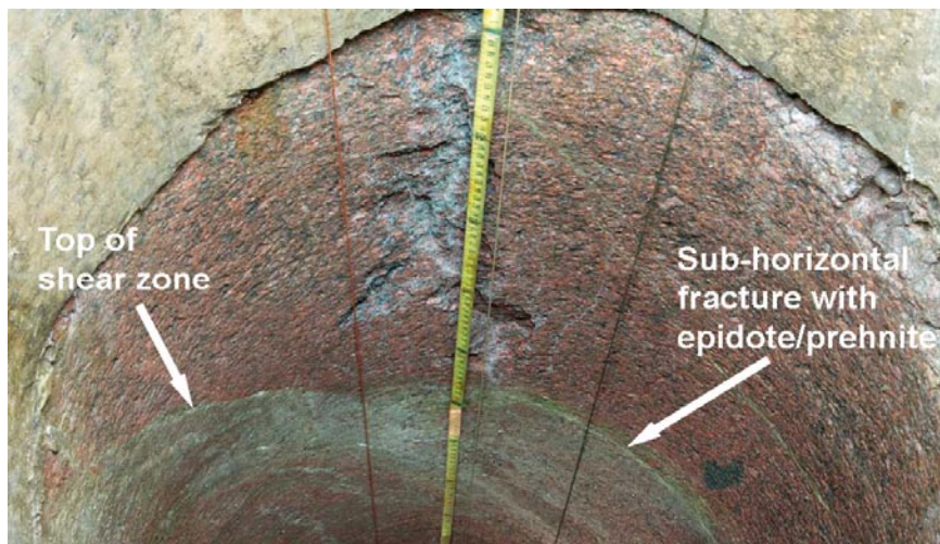
Figure S-2. Observed spalling in heating hole KQ0046G04 on the same side as in Figure S-1. The top of the shear zone to the left cuts through the borehole down to the southeast. An epidote/phrenite filled cataclastic structure runs sub horizontally across the borehole. The latter is cut by the shear zone.
