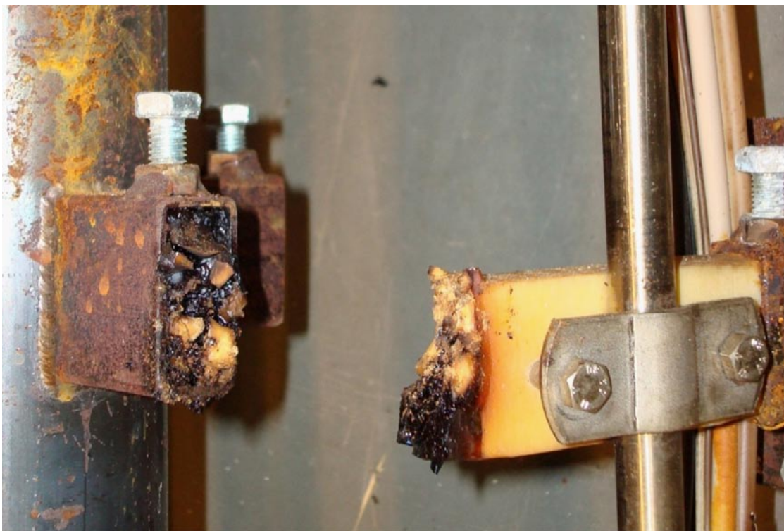
Figure 5-1. Photograph of one of the spacers used in the first heating test. The spacer of polyurethane became too hot and started to melt (Photo R Glamheden).
