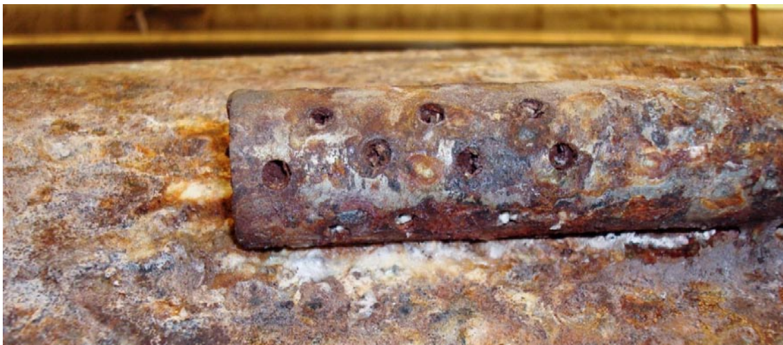
Figure 5-4. Photograph of the perforated part of the tube of the lower RH-gauge after removal of the test equipment in Test 3. The perforation was clogged due to substantial corrosion during the test (Photo R Glamheden).
