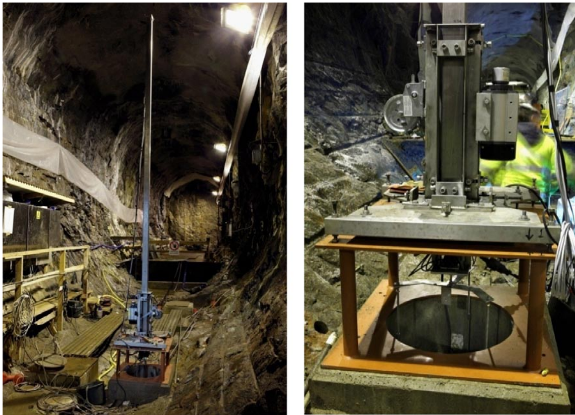
Figure 7-1. Lifting device for documentation of the spalled notch in the heating holes.
