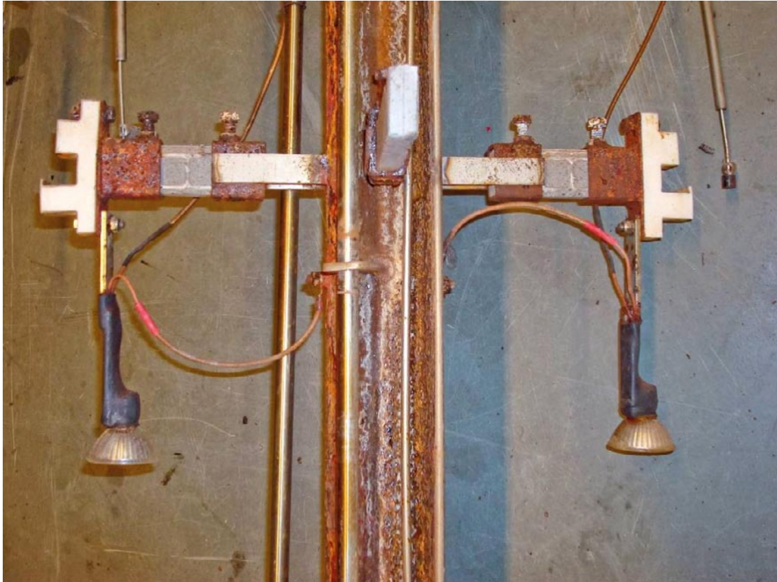
Figure U-8. Shows the state of the holder after completion of Field Test 2.
