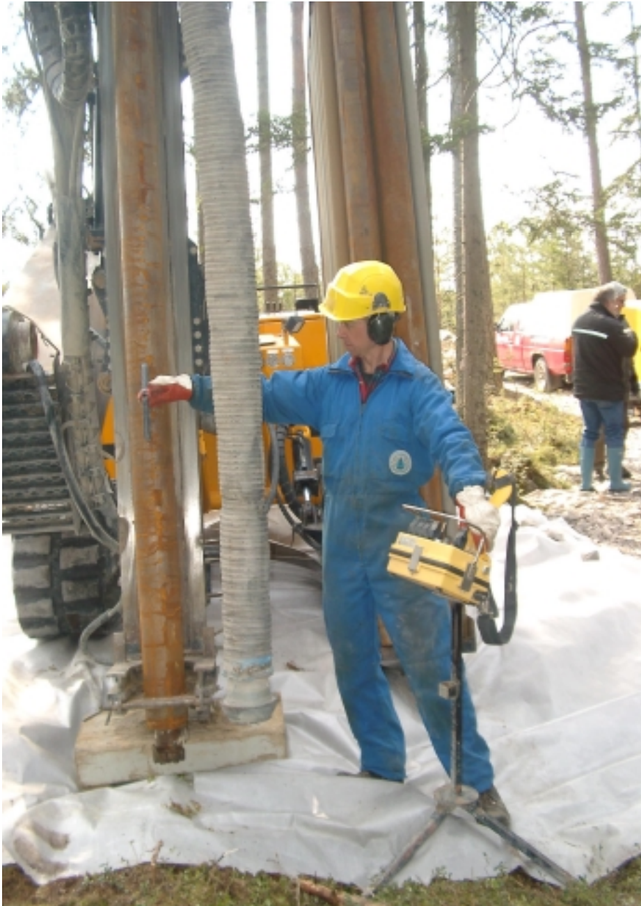
Figure 3-2. The Nemek 407 percussion drill machine with a 168/160 mm temporary steel casing simultaneously driven through the overburden and approximately one metre into the bedrock while drilling. Photo by Alf Sevastik.
