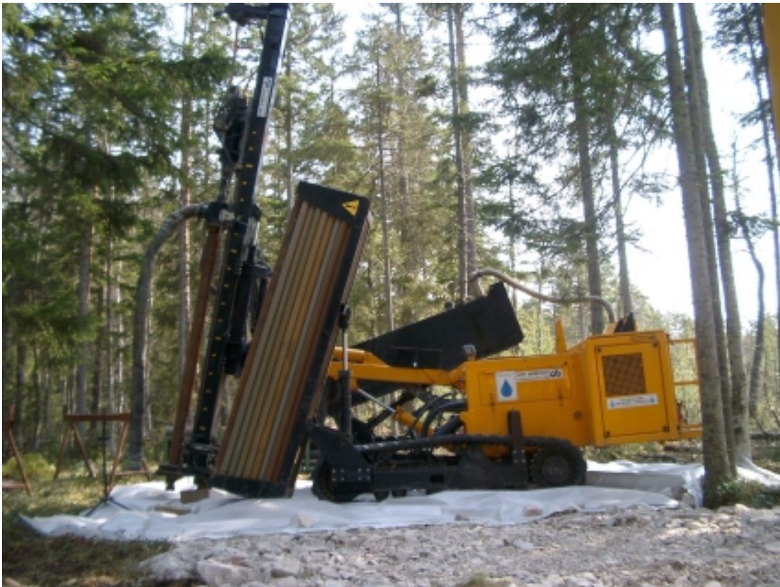
Figure 3-1. The Nemek 407 percussion drill machine engaged for drilling the three monitoring wells in unconsolidated soil layers at drillsite DS1. Note the fluidproof cover beneath the drill rig used for protection of the ground in case of unintentional oil spillage. Photo Alf Sevastik.
