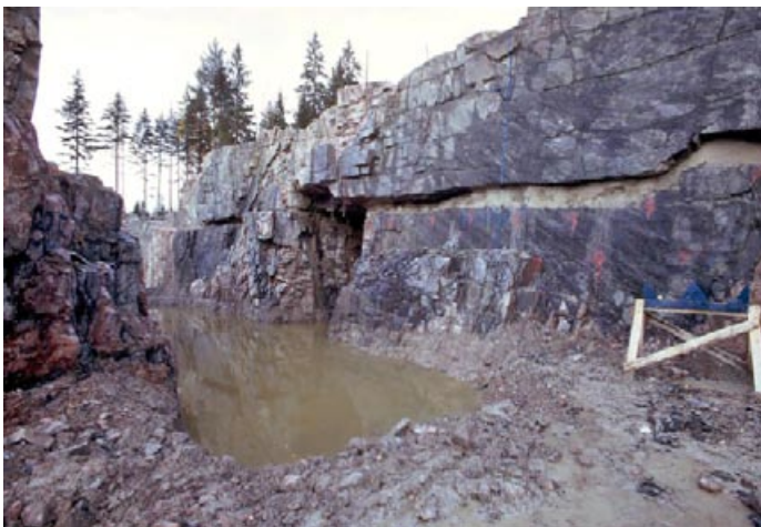
Figure 7-21. Example of a horizontal sediment-filled fracture at Forsmark, which was exposed during the construction of the nuclear power plant in the 1970s. From /Leijon 2005/.
