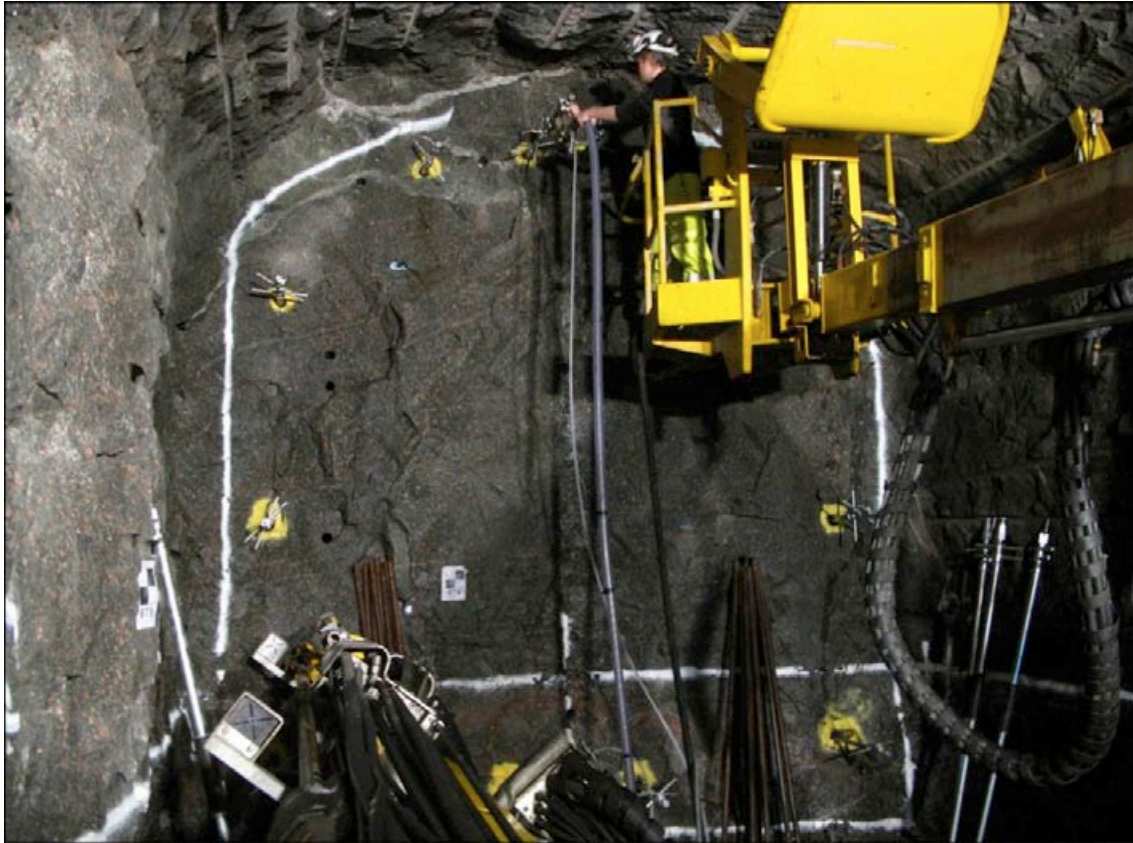
Figure 5-6. A performed grouting fan inside tunnel contour, photo from SKB:s sealing project at great depth.
