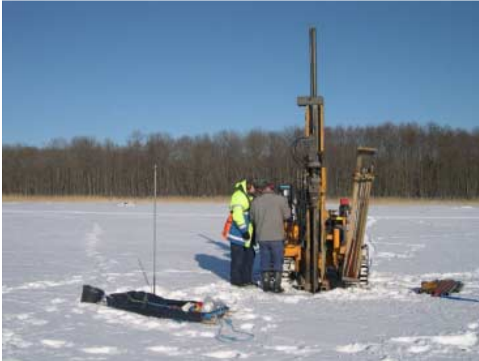
Figure 4-1. Illustration of work with groundwater pipes, running parallel with ongoing investigation of the sedimentary sequence, at the drill site SFM0043/SFM0025. The rod on the left hand side of the drilling machine is located in the borehole to mark the position of the coring site.
